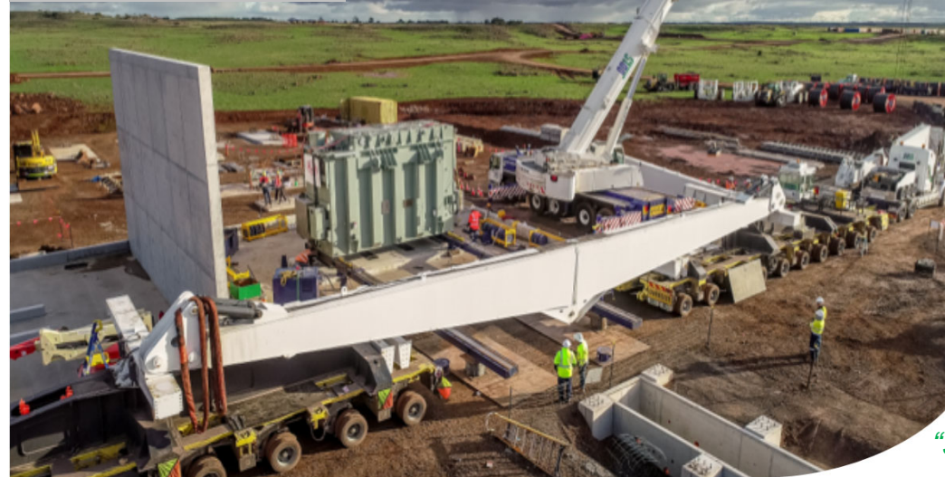
33/220kV, 240MVA Transformer
