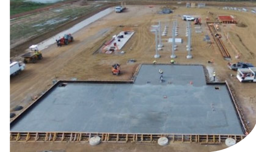
Bluegums 500/220kV substation
