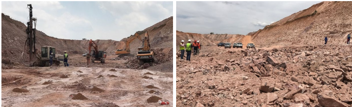
Image 2: Pit 3's successful trialling of Nonex in December 2018 provided production efficiencies and significantly decreased breakdowns of the Excentric Rippers
