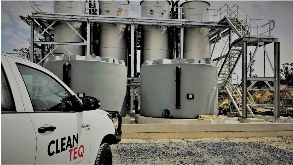
Clean TeQ plant installation at Fosterville Gold Mine, Victoria
