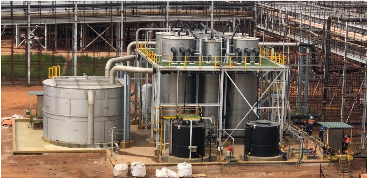
Clean TeQ Continuous Resin-In-Column Ion Exchange plant in DRC
