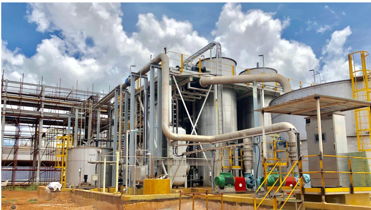
Clean TeQ Continuous Resin-In-Column Ion Exchange plant in DRC
