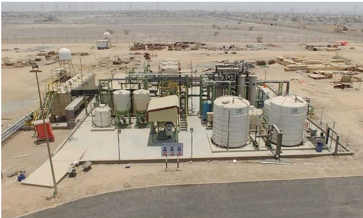
Clean TeQ CIF® plant constructed and awaiting commissioning in Oman
