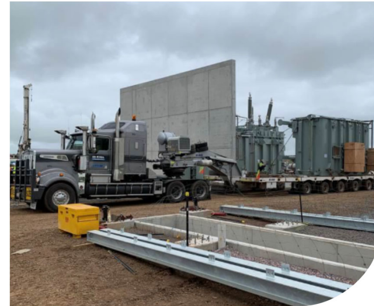
Installed wind farm transformers
