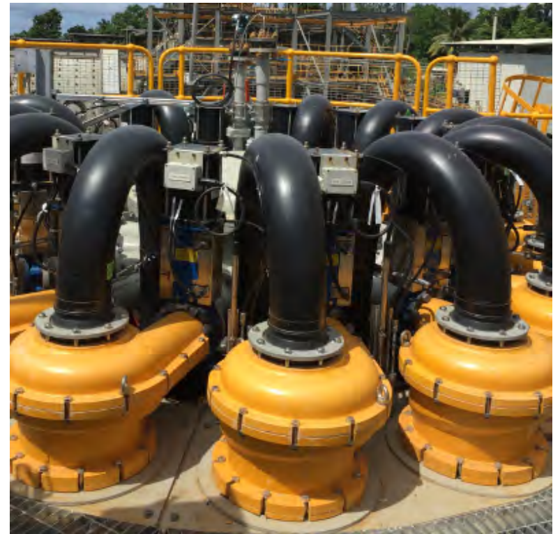
Float Tails Leach cyclone pack
