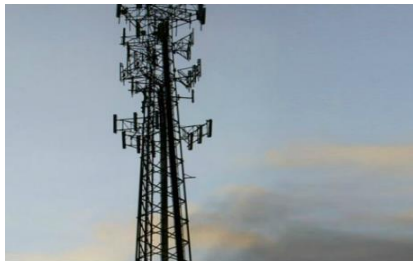
Mobile Phone Tower Crown Castle International Corp (US) Mkt Cap (July 2020): A$98 billion
