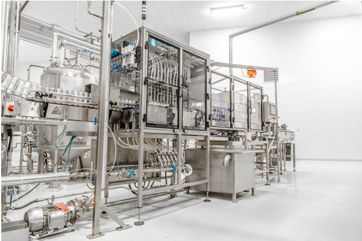
Image 2 – Canned beverages equipment at the Peak Processing facility
