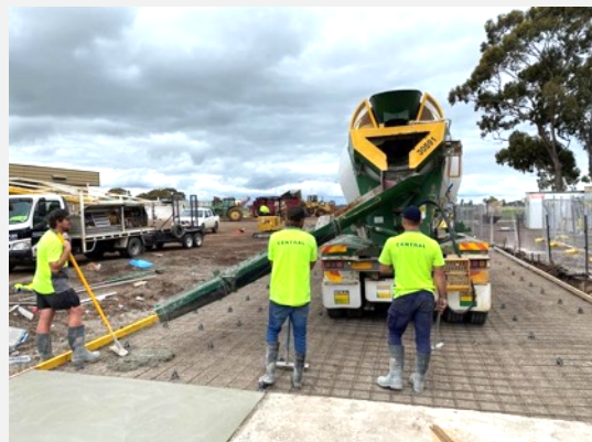
Photo, above: Central concreting finishing off the new roadway to allow trucks to more easily enter and exit the lignite storage area.
