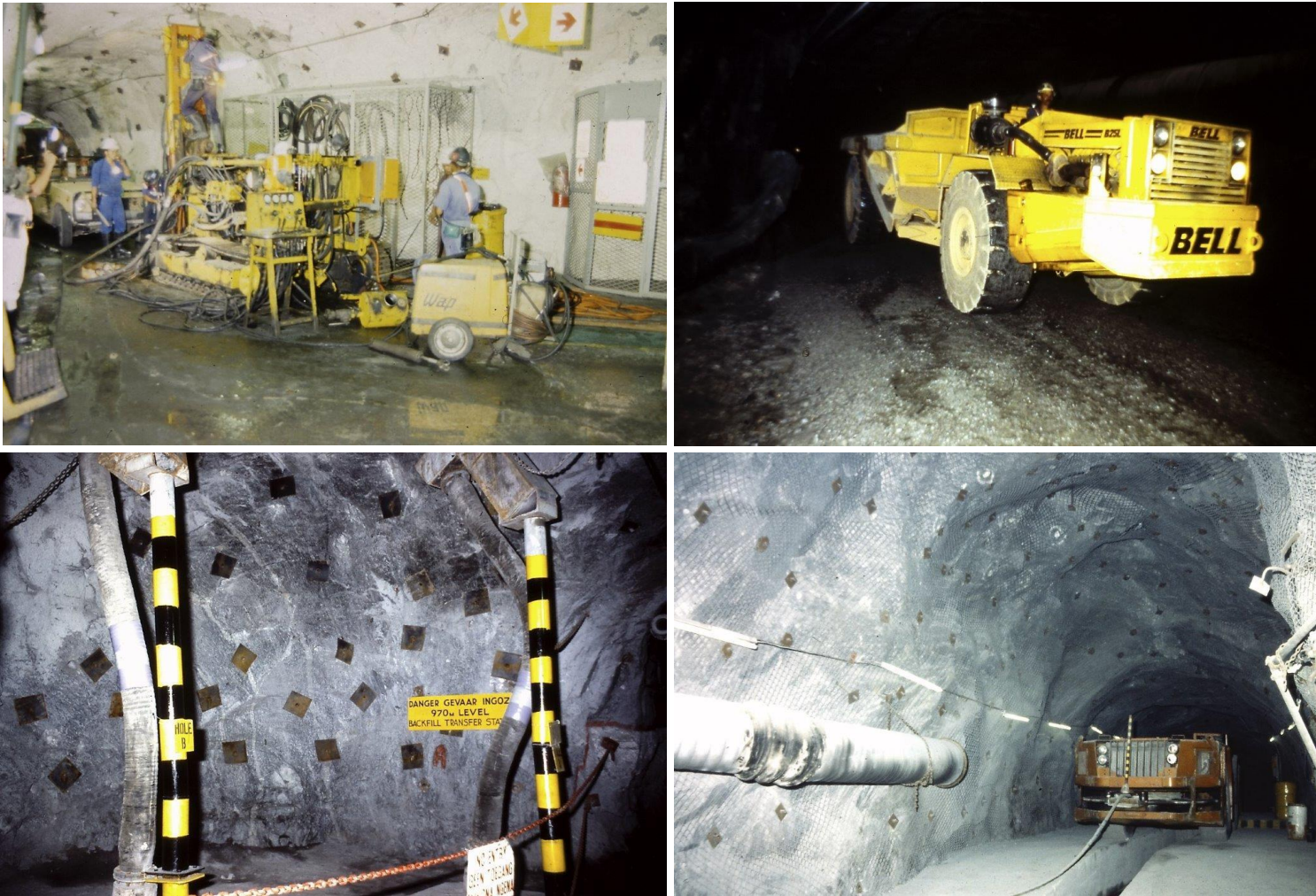
Figure 5: Historic underground mining activities at the Nigramoep and Carolusberg mines, showing the extensive underground development and infrastructure in place.
