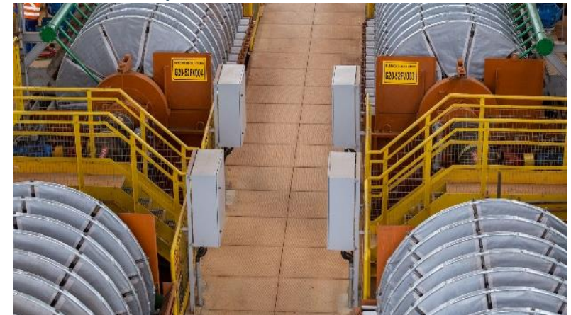
Samarco filtration plant
