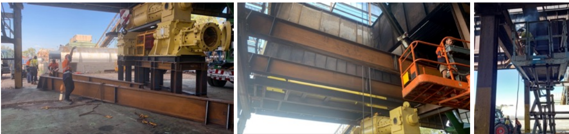
Above: installation of mixer structural support beams above the mill and extruder.
