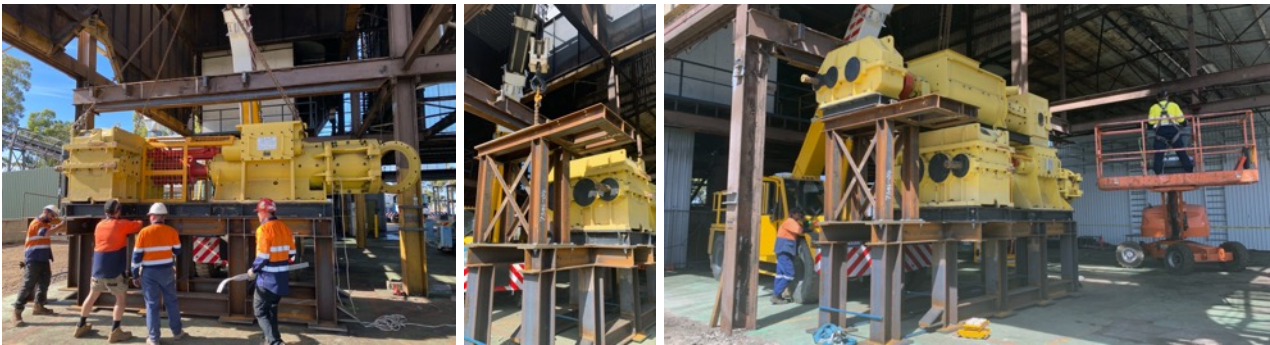
Above: positioning and fastening of the extruder, followed by installation of mill and mill support structure.
