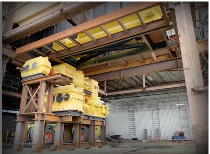
Coldry Primary Processing Train Foreground: mixer, mill and extruder. Background: Cable trays installed ready for Motor Control Centre to be installed.
