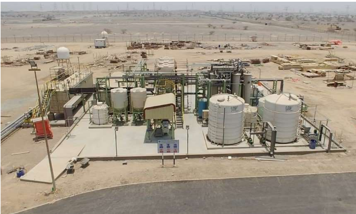
The Company's proprietary DESALX® (two-stage CIF®) plant in Oman
