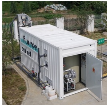
Aspiral S1 near homes, Hefei, Anhui province
