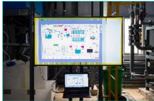
Control console manages remote, automated plants
