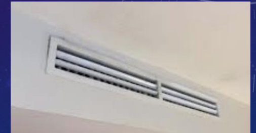
Supply air grill
