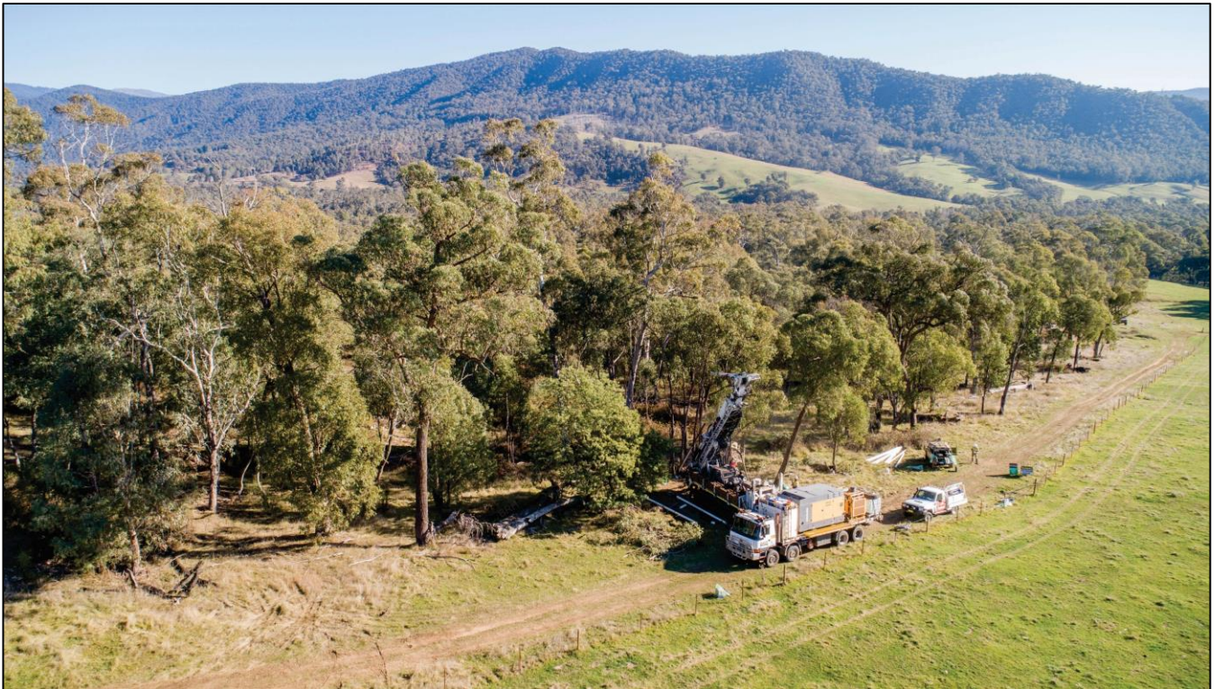
Figure 4: Photographs of Durock Drilling Pty Ltd setting up on the first hole of the 3,500m program.
