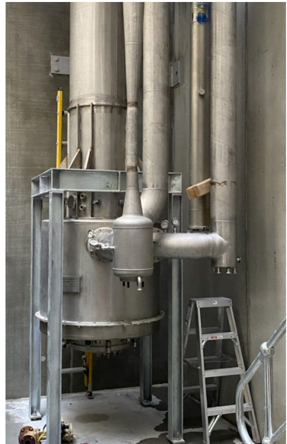
Image: Piping and services
