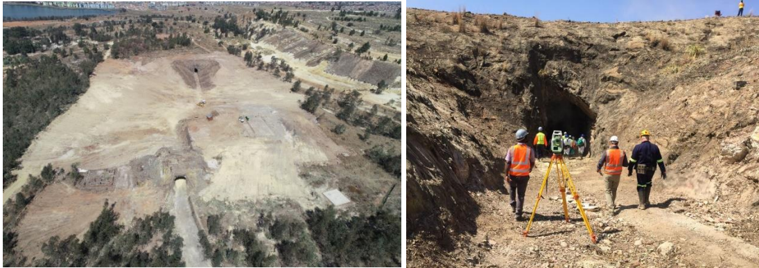
Image 4: (Left) Qala Shallows Site Preparation and (right) Technical Team Site Inspection at the Qala Adit
