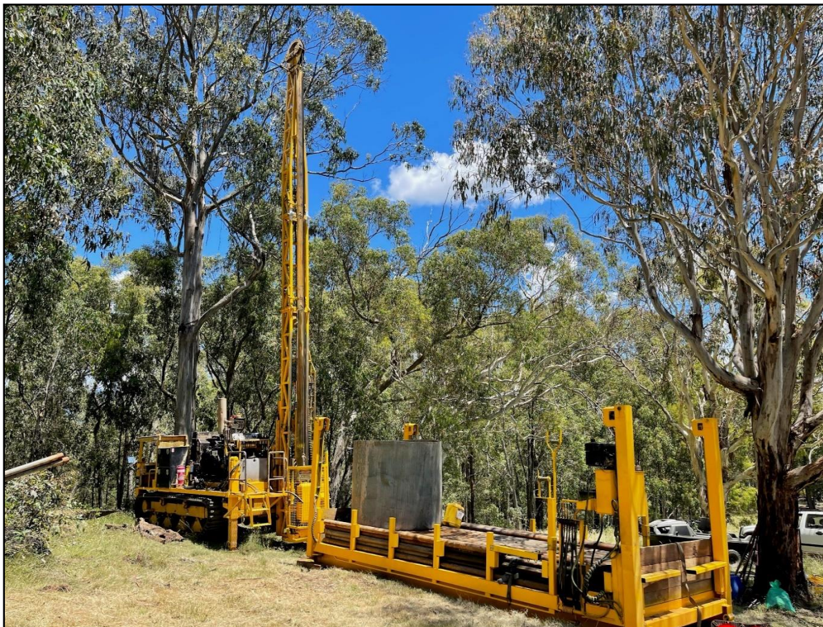
Figure 1 – Territory Drilling set up on hole EMDDH006 at Granite Flat, targeting a geophysical anomaly ~350m below surface (see figure 2).
