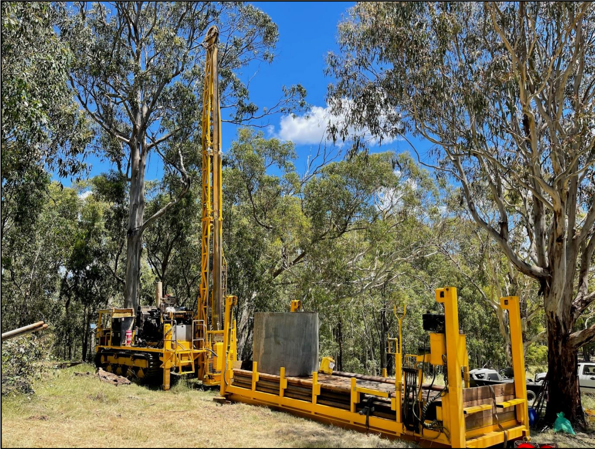
Figure 1 – Territory Drilling set up on hole EMDDH006 at Granite Flat, targeting a geophysical anomaly ~350m below surface (see figure 2).
