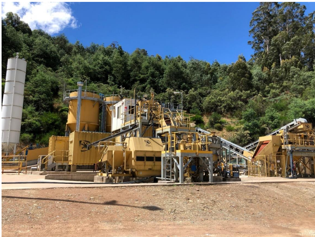
Figure 1: Gold processing plant at White Rock’s Morning Star Gold Mine, NE Victoria
