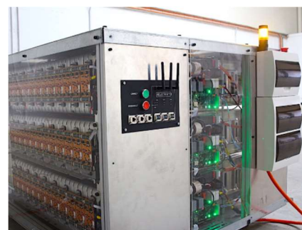
Battery Energy Storage System (BESS) made with EV cells
