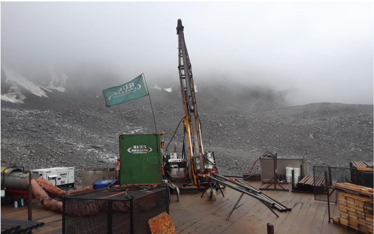
Figure 1. Rig mobilized at Cathedral to test the potential Korbel Main feeder system
