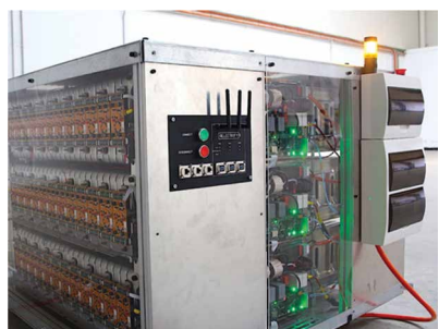
Battery Energy Storage System (BESS) made with EV cells
