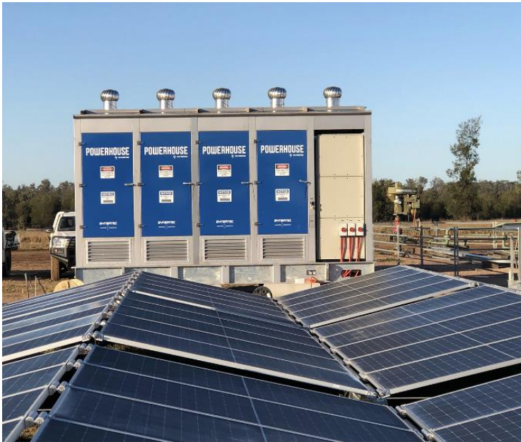
Figure 1: Powerhouse in operation during site acceptance testing.
