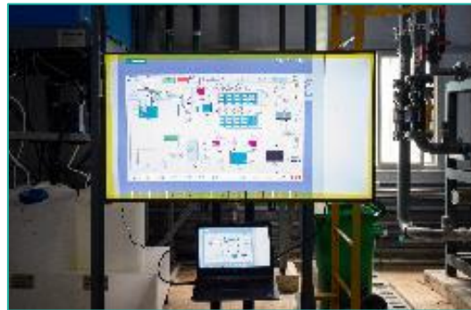
Control console manages remote, automated plants
