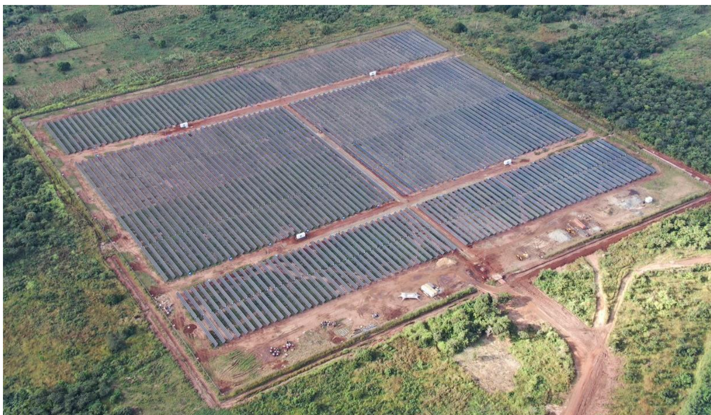
Figure 1: Balama Solar & Battery System.
