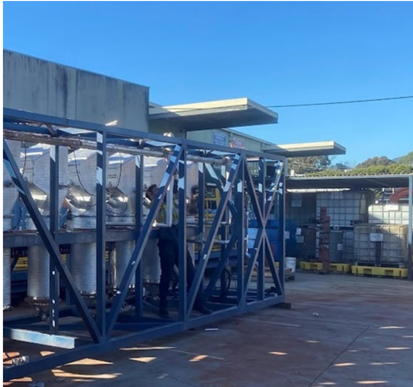
Go2Lithium demonstration plant – Adsorption skid
