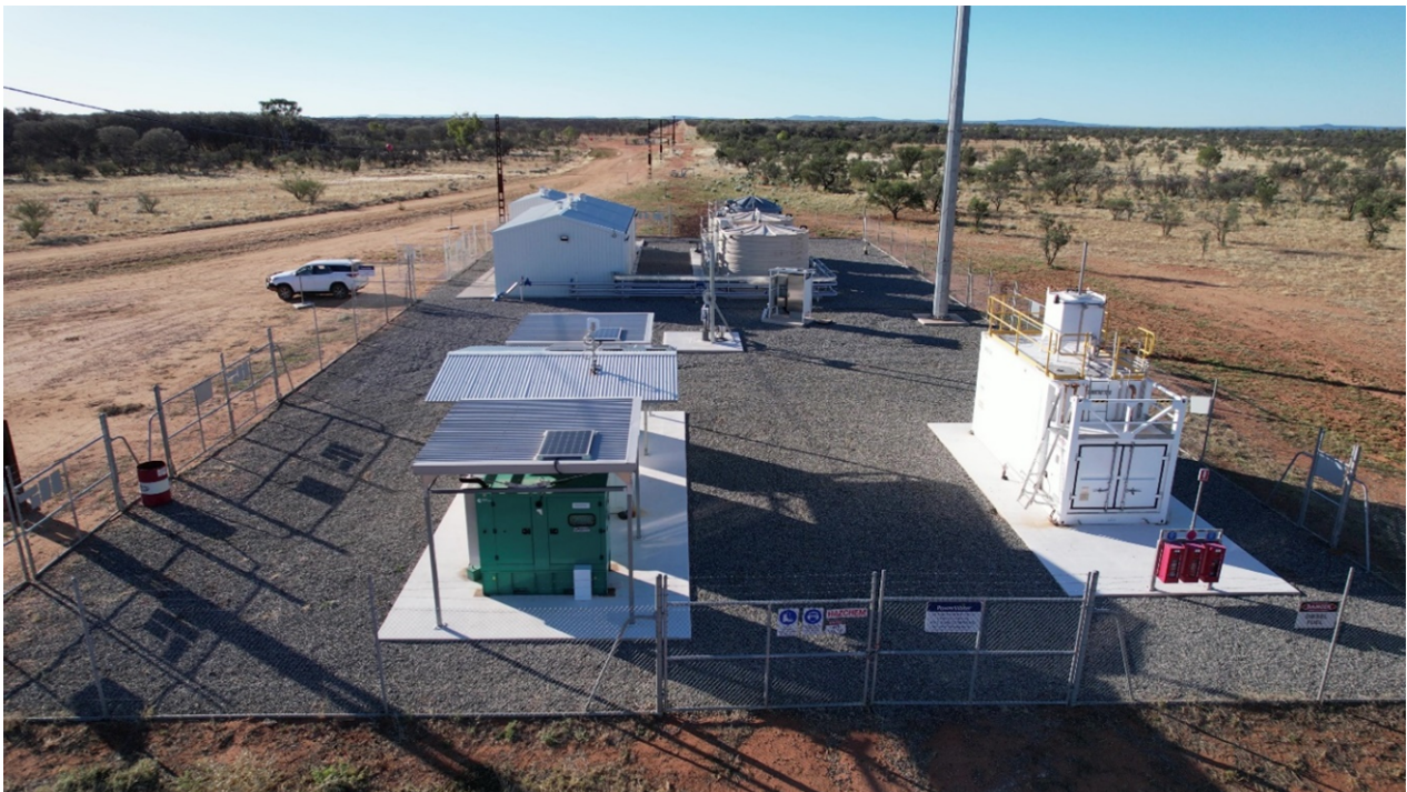
Photo of the Laramba Water Treatment Plant in Remote NT
