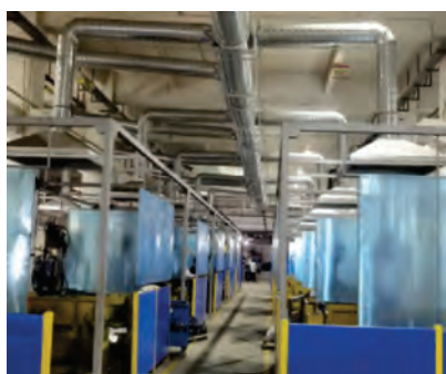
Newly installed weld fume and dust extraction system at an APG supplier
