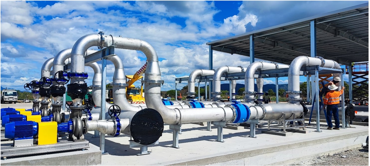
Photo of the Townsville plant showing pumps and UV disinfection units
