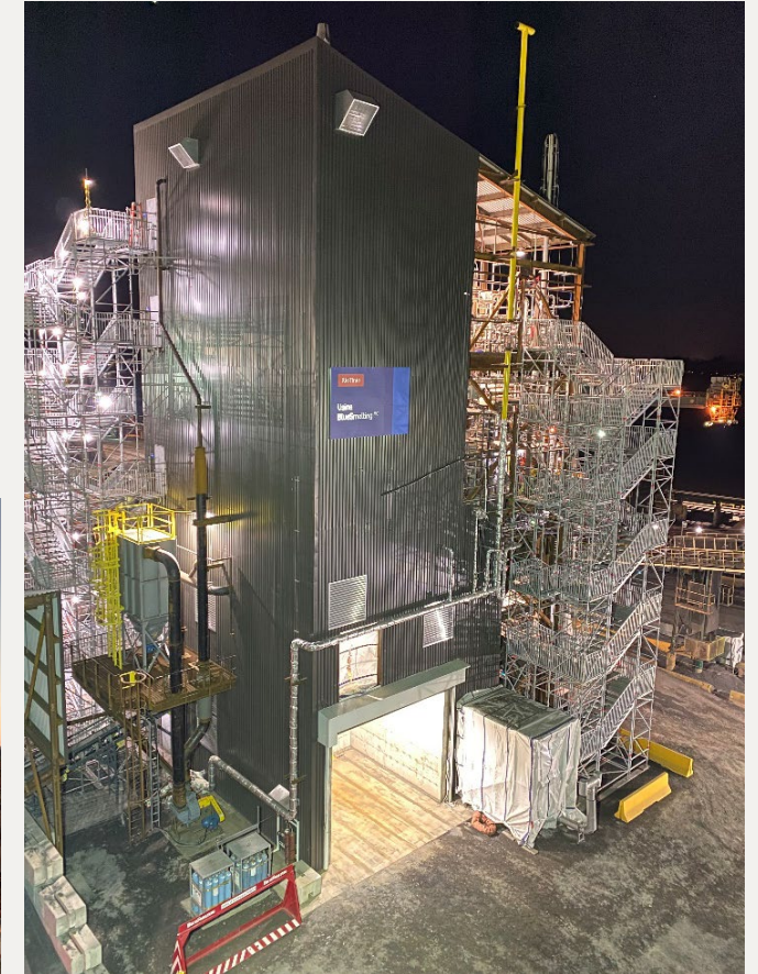
RTIT BlueSmelting™ demonstration plant
