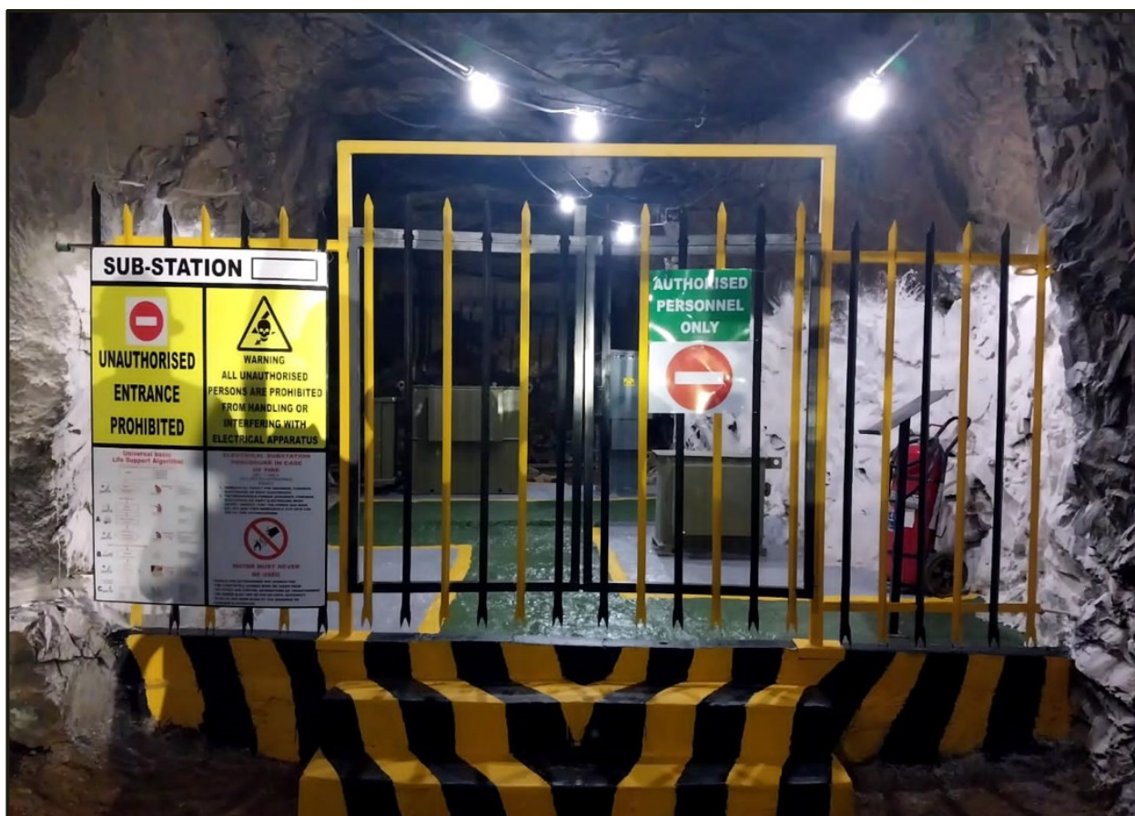
Photo 1: Underground Electrical Substation.
