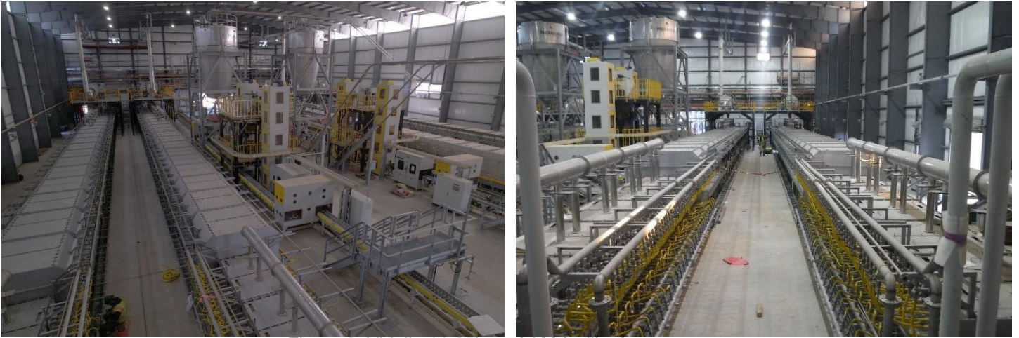
Figure 6: Vidalia 11.25ktpa AAM facility furnace area.
