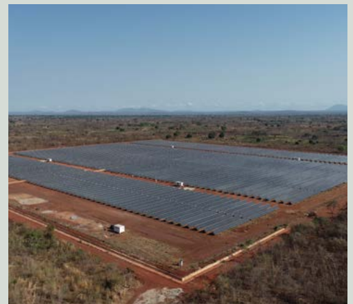
▲ Balama solar and photovoltaic array
