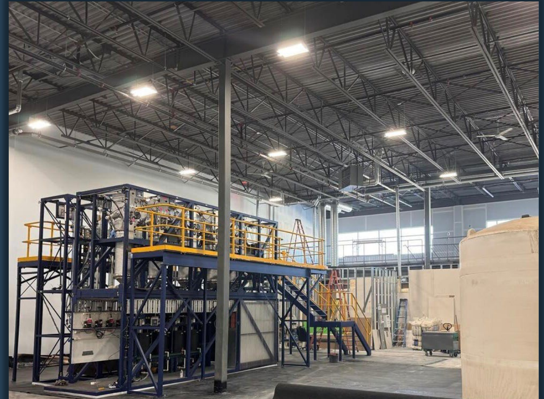
Clean TeQ cDLE ® Pilot Plant being installed at the LithiumBank Facility in Calgary
