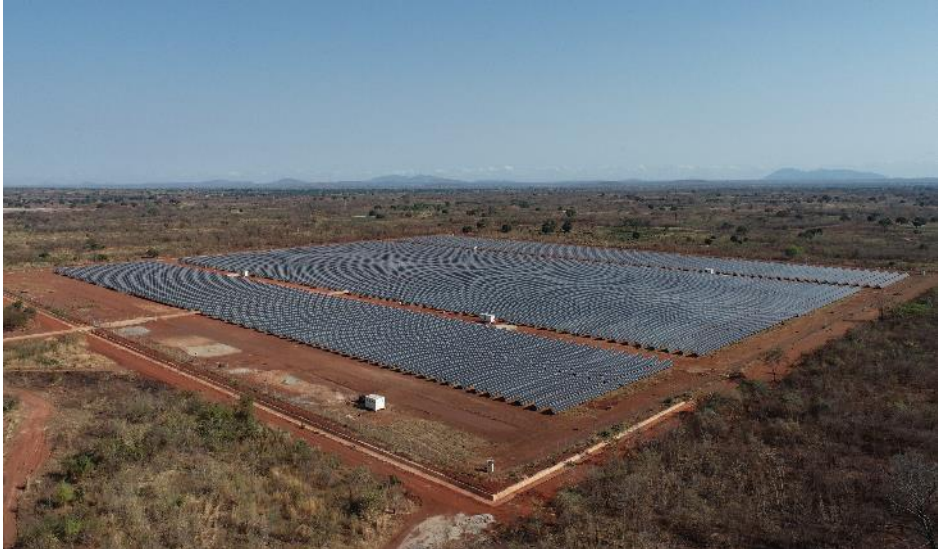
11.25 MWp solar photovoltaic array
