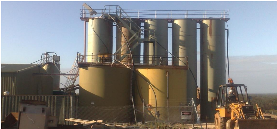
Carbon in Leach (CIL) and Carbon in Pulp (CIP) tanks
