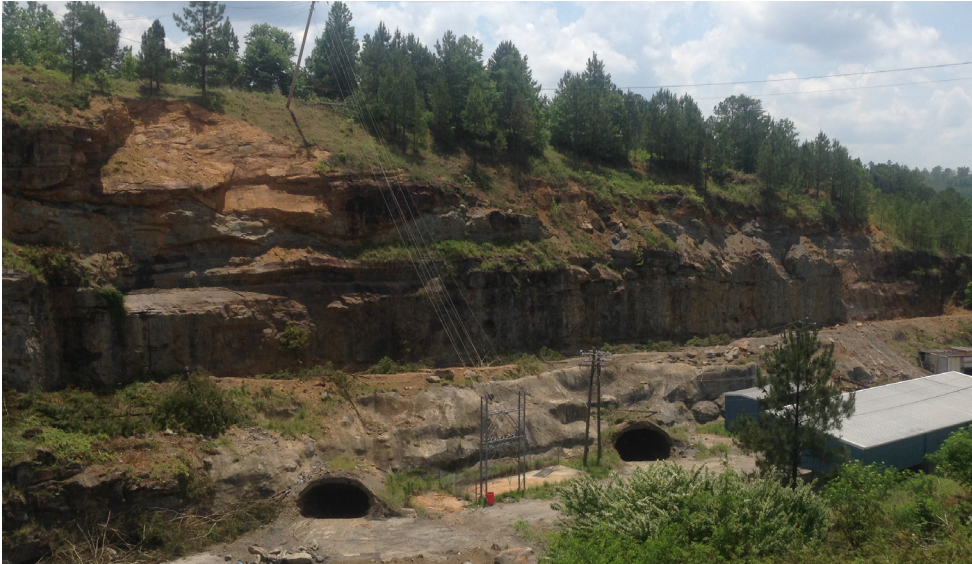
Figure 1: Site works have been undertaken to enable re-opening of the portals in accordance with MSHA standards
