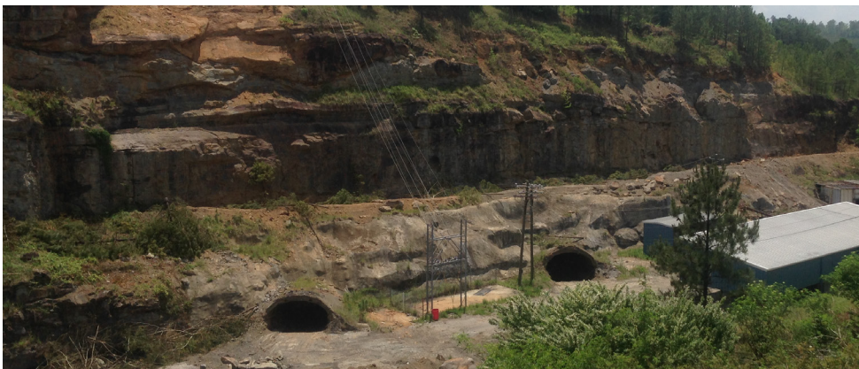
Figure 1: Site works have been undertaken to enable re-opening of the portals in accordance with MSHA standards
