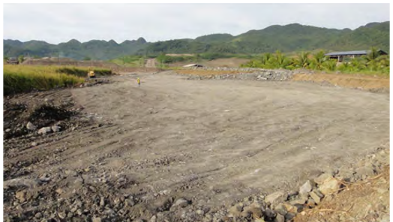
First lift of rockfill after 3 full shifts of fill placement, ~8,000m 3 of rockfill to date.
