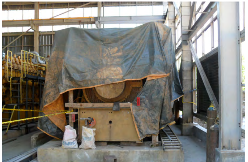
New 2MW Genset in position ready for connection.
