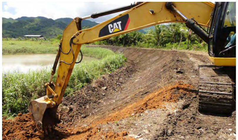
South embankment upstream face stripped of grass and topsoil to prepare for fill placement on the beach.
