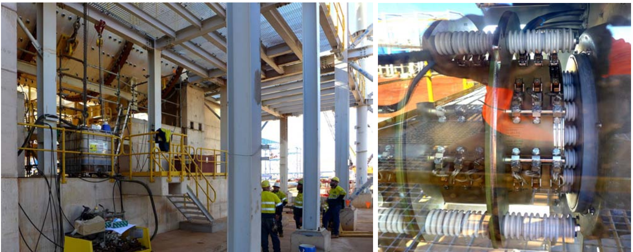
Figure 11: Pipe-bridge structure (top image); Ball Mill lining being installed (middle image); pre-start meeting at Ball Mill (bottom left) and shielded high-voltage transformer at the Ball Mill drive train (bottom right)
