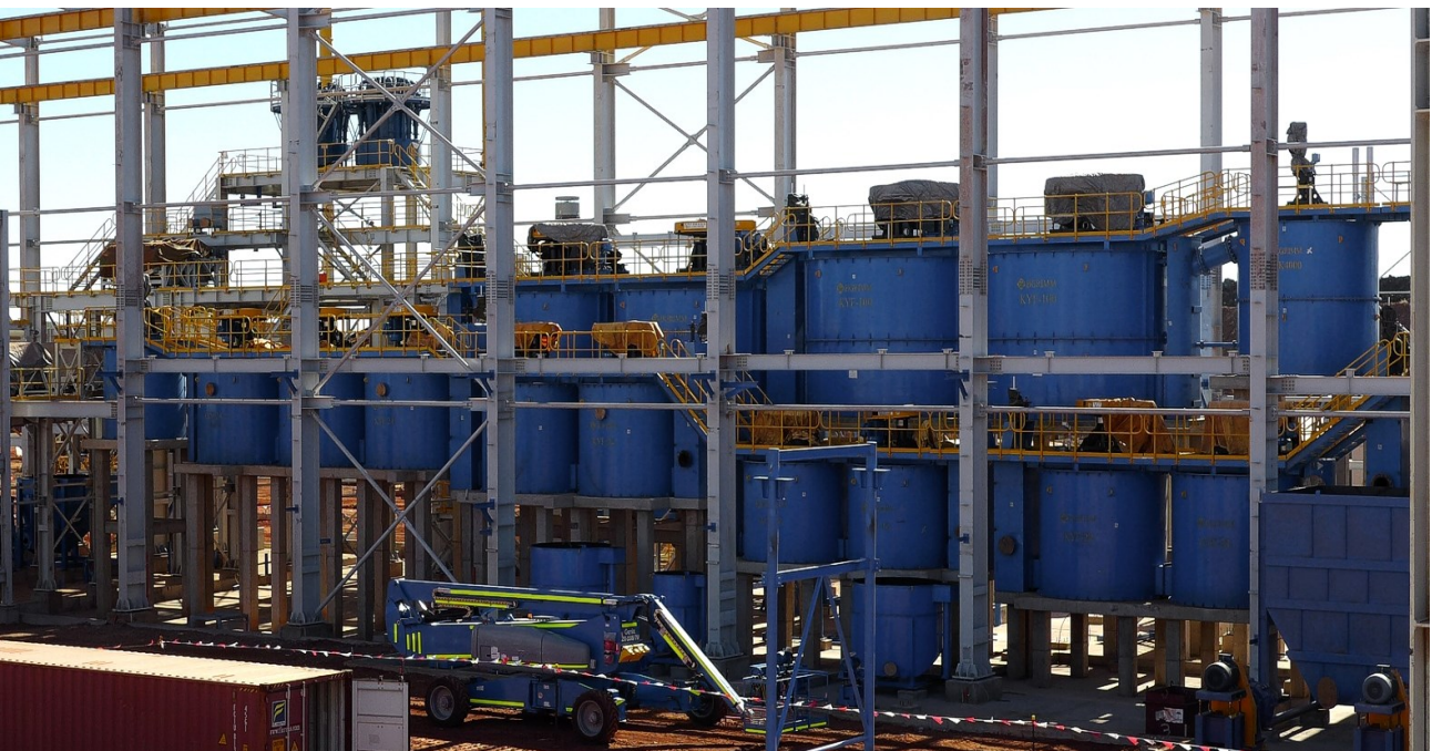
Figure 14: Flotation Cell building - low-pressure air blowers (top) and copper and cobalt float circuits (bottom)
