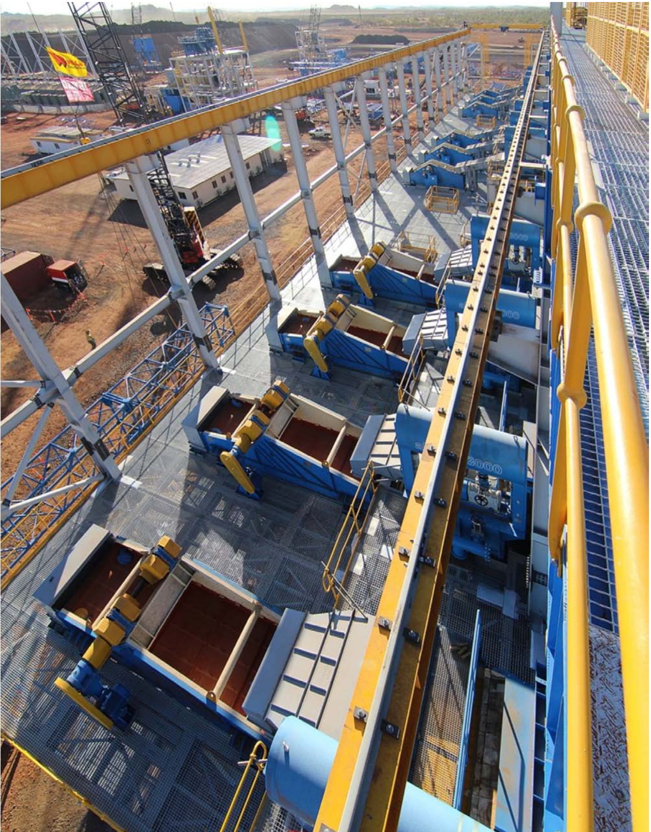
Figure 3: Gravity Jig Building (looking west) - continuous alljig® units fade into the distance on level 3
