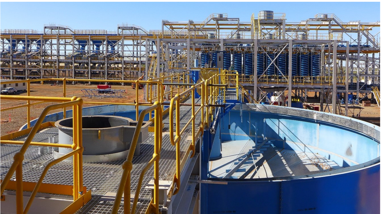
Figure 17: Top image shows Scrubber Circuit and bottom image shows the Gravity Jig building (far background), Spirals (middle distance) and copper concentrate thickener tank as viewed from the Thickener/Filtration circuit (foreground).
