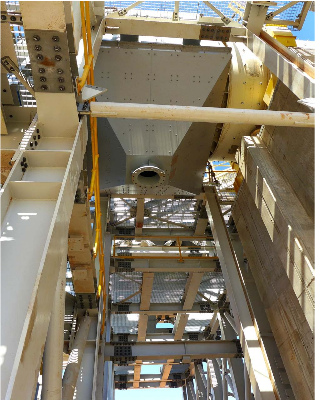
Figure 19: Scrubber discharge sump
