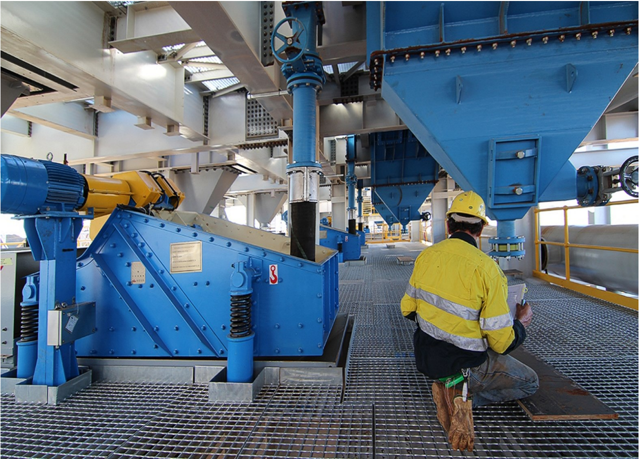
Figure 6: Gravity Jig building - fines screen (left) and jig hutch (base of jig) on right.
