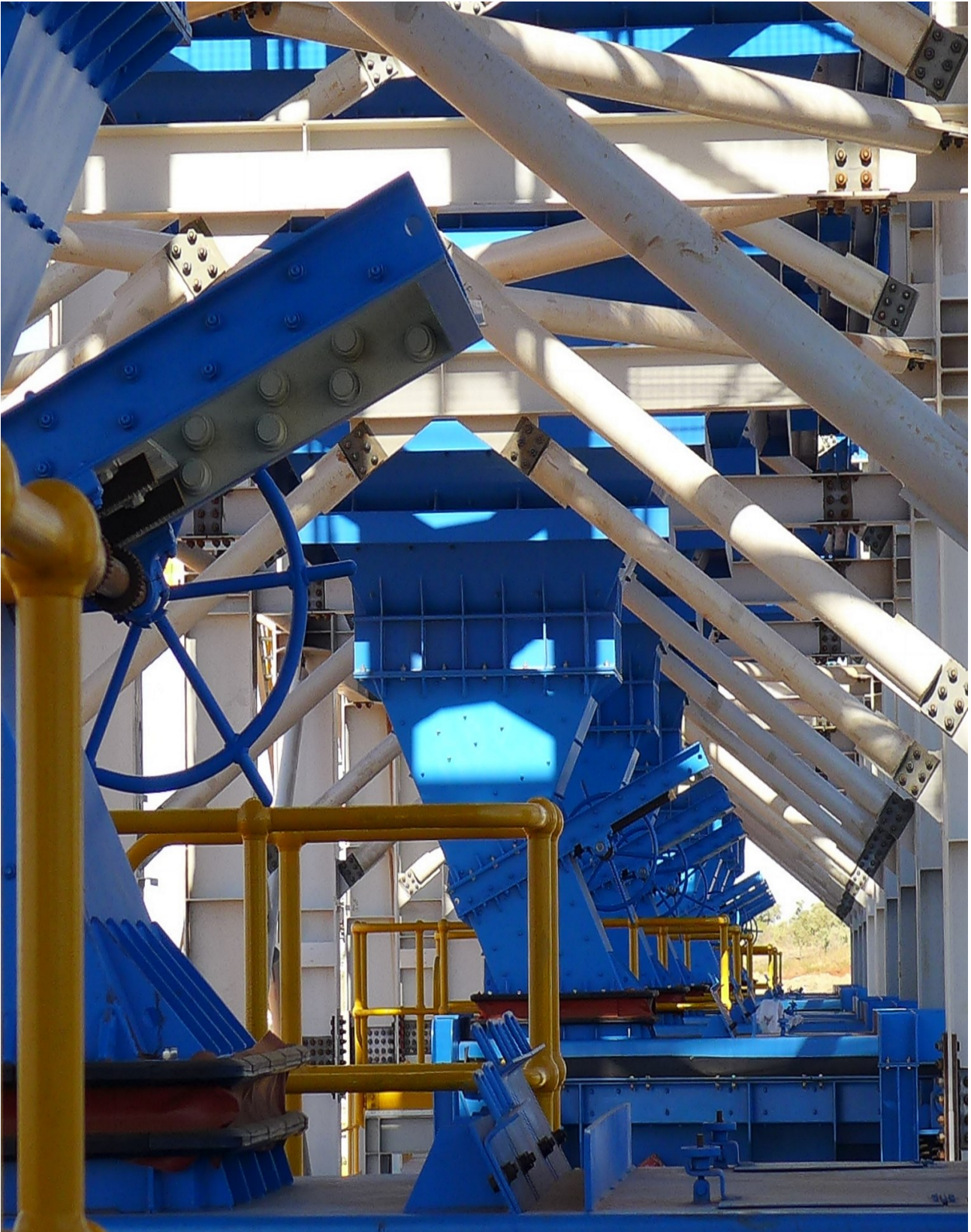
Figure 21: Gravity Jig Building - level 2 Jig-feed chutes and bank of continuous alljig® units.
