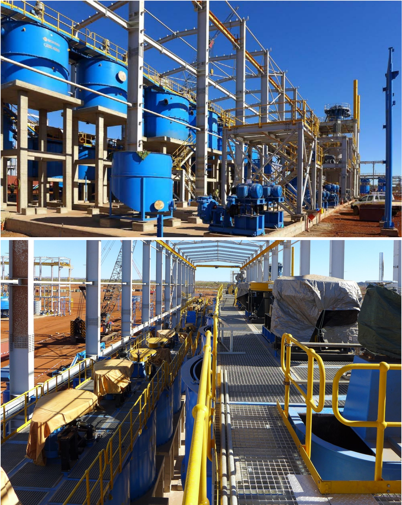
Figure 13: Flotation Cell building - flotation cells (top) and cell agitators (bottom)
