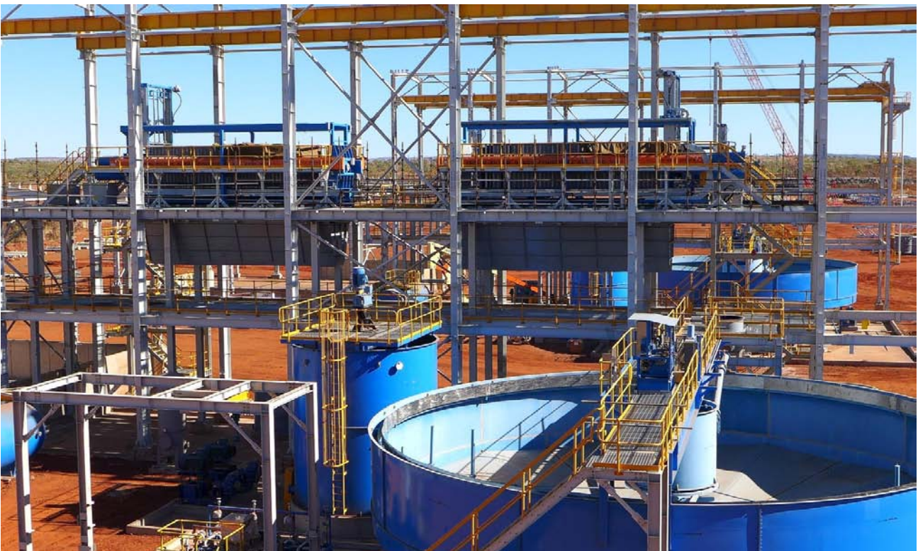
Figure 16: Thickener/Filtration circuits viewed from the Flotation Cell building (top image) and; Thickener/Filtration circuit up close.
