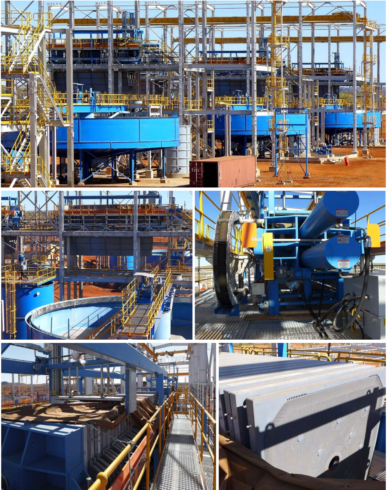
Figure 18: Thickener/Filtration circuits (above) and close up of filtration unit and panels (bottom images)
