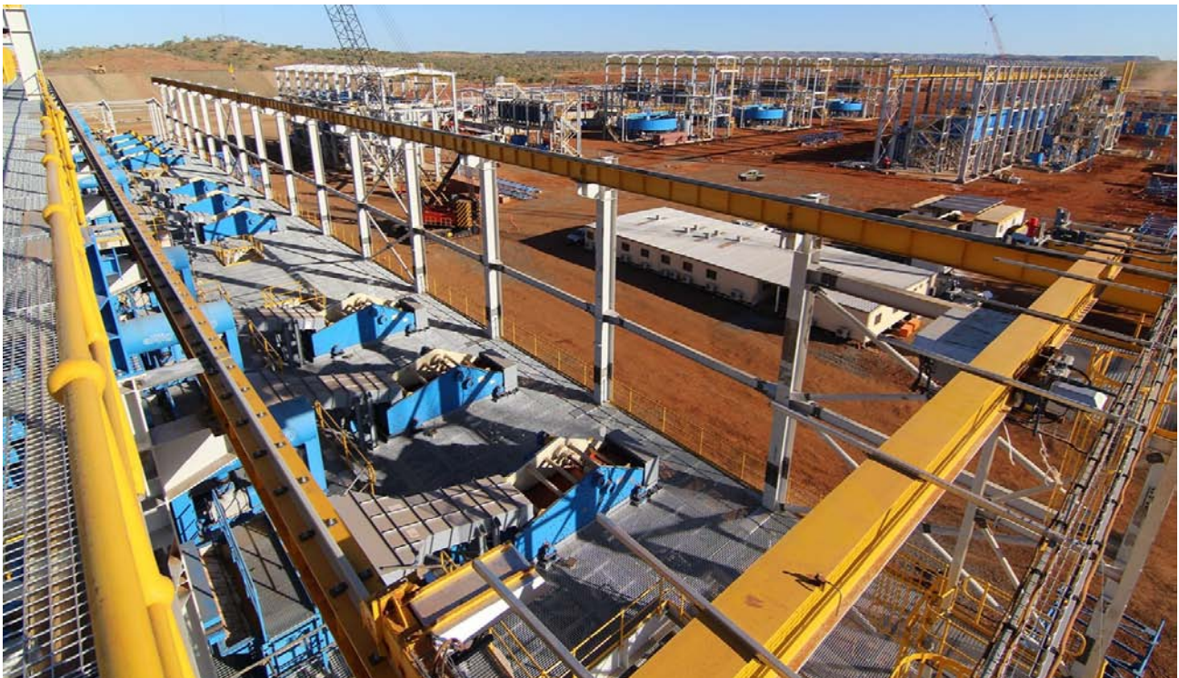
Figure 4: Gravity Jig Building - looking east; continuous alljig® units fade into the distance on level 3. From left to right in background; Table Separator Circuit; Spiral Separator Circuit; bank of three Thickener/Filtration Circuits; Flotation Cells; Cobalt Re-grind Circuit and; Magnetic Separation Circuit.
