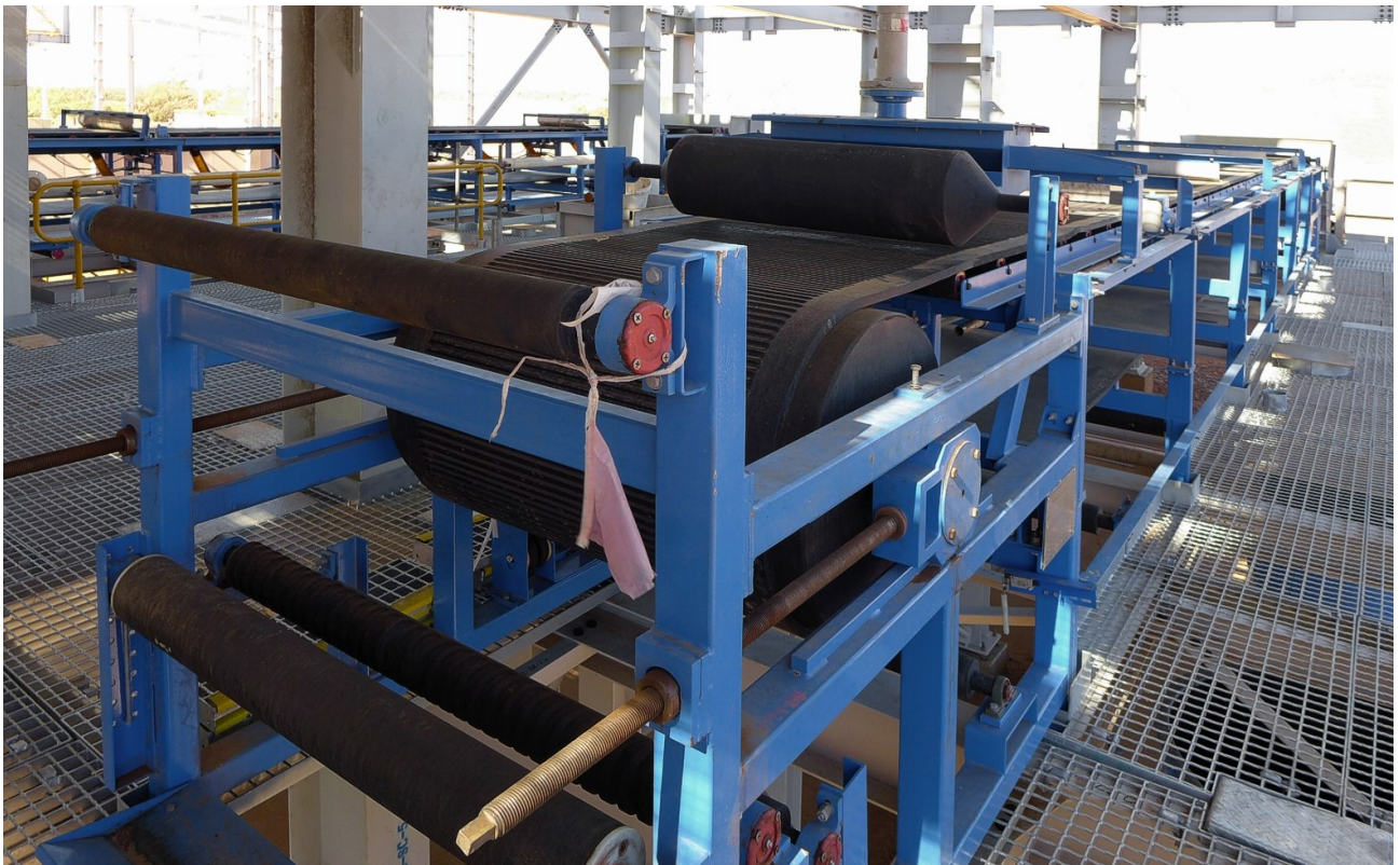
Figure 20: Table Separator Circuit building (top image) and close up of vacuum belt filter (bottom image)
