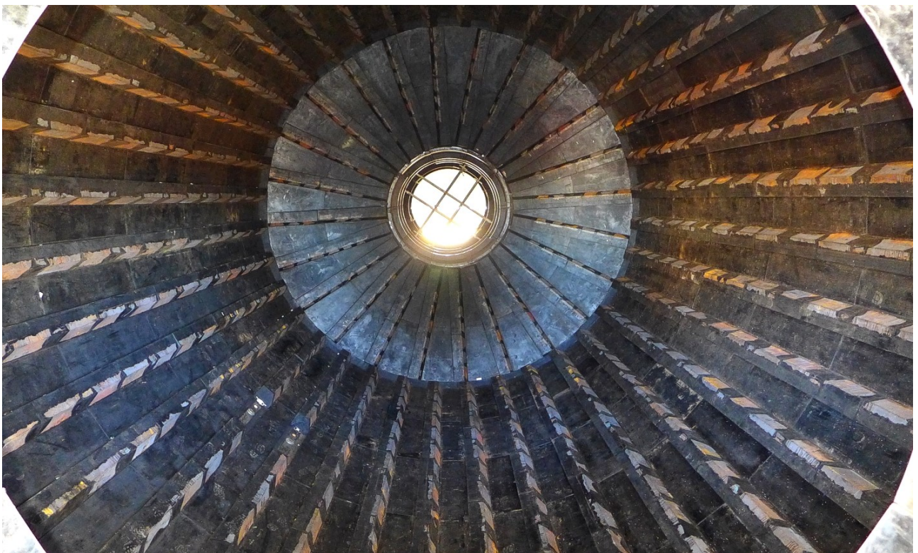
Figure 12: Ball Mill discharge trommel (top image) and high-impact poly-met lining of Ball Mill almost complete (bottom image)
