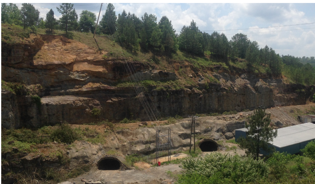
Figure 3: Site works have been undertaken to enable re-opening of the portals in accordance with MSHA standards
