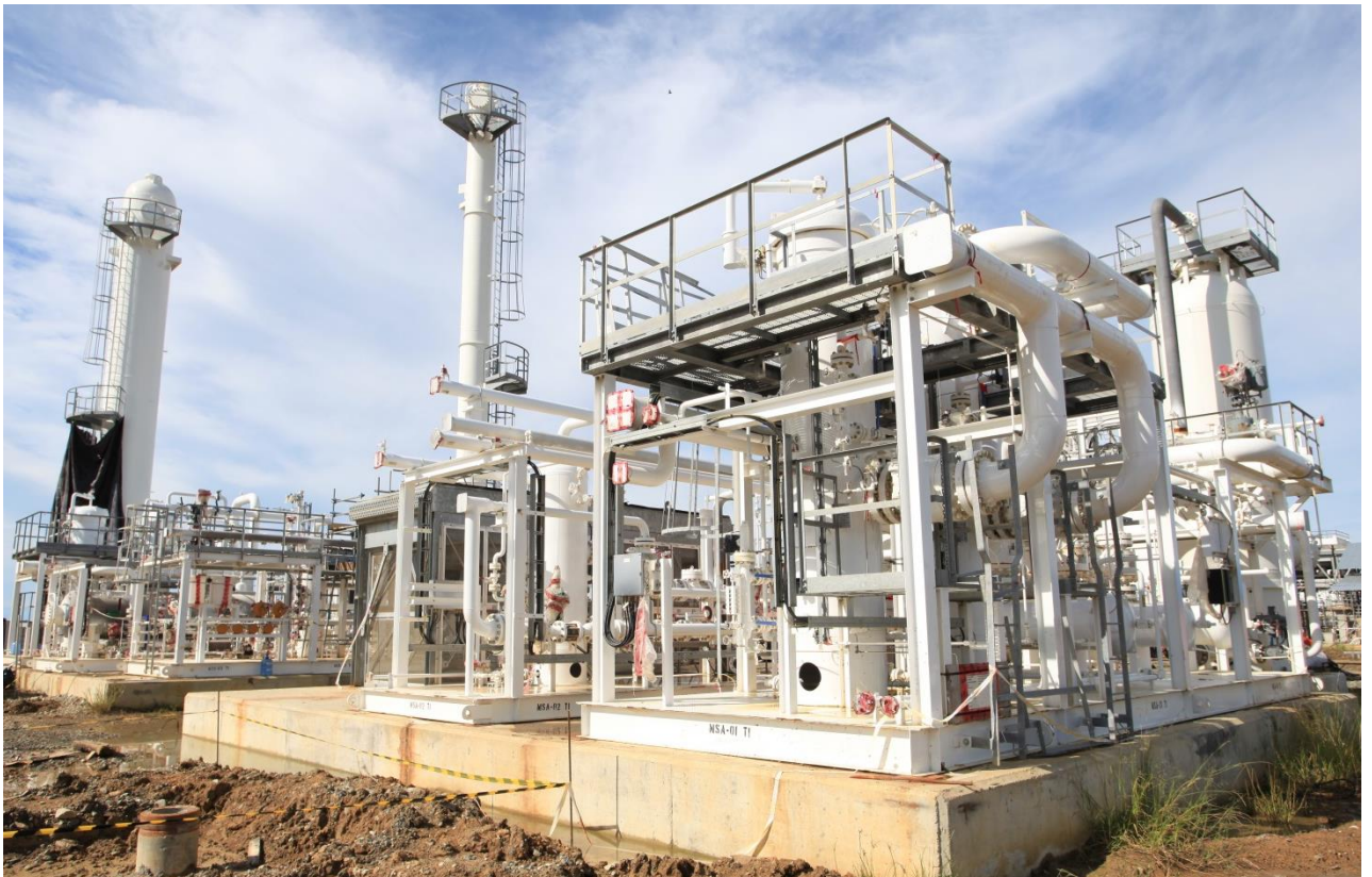
Main Processing Plant Area – Pre-treatment Plant of MPA I
