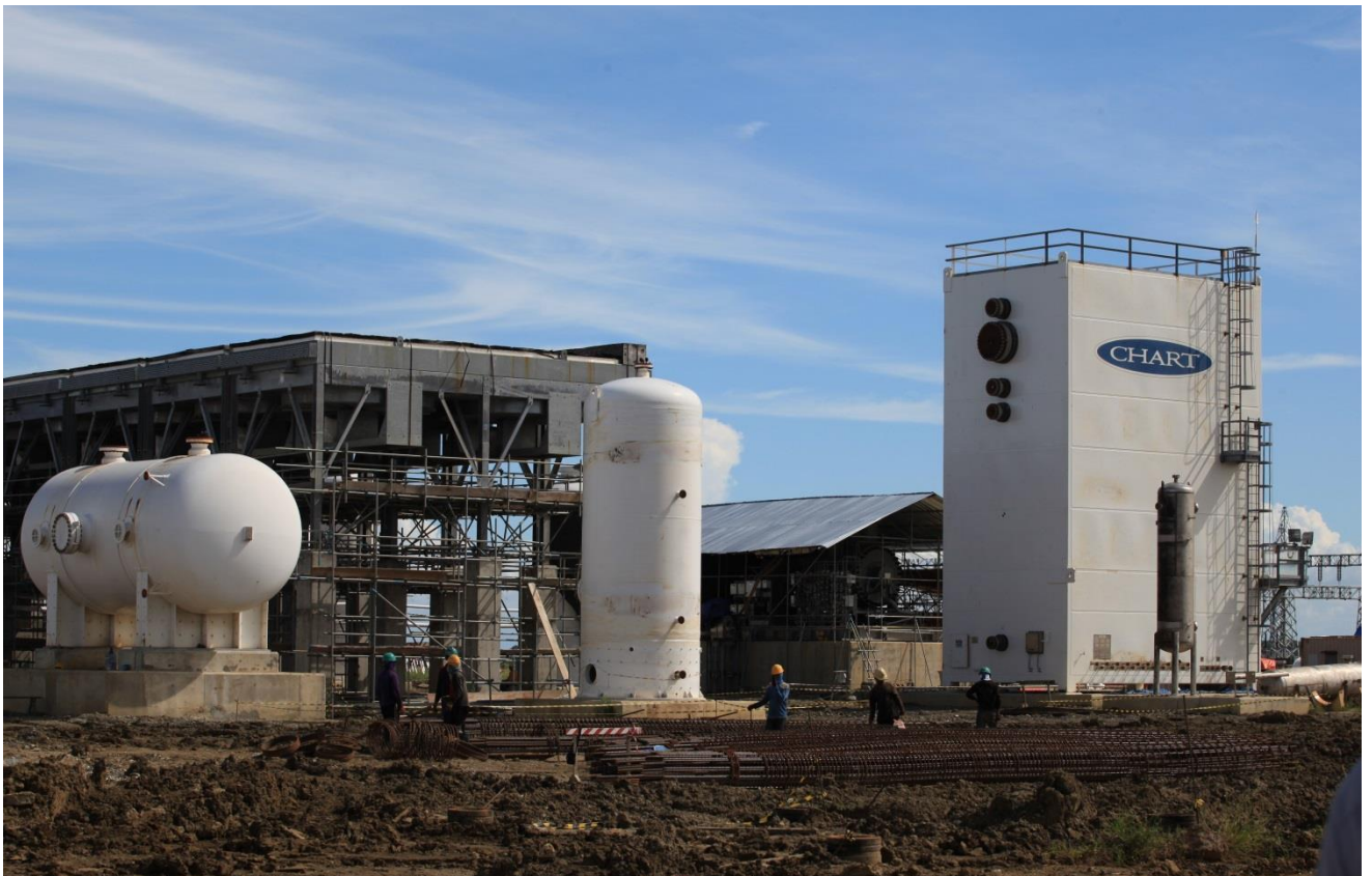
Main Processing Plant Area – Phase I
