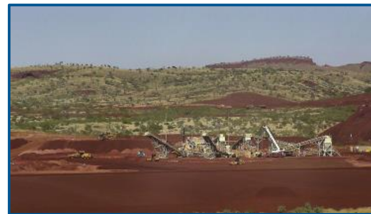
Iron Valley Commissioning - August 2014
