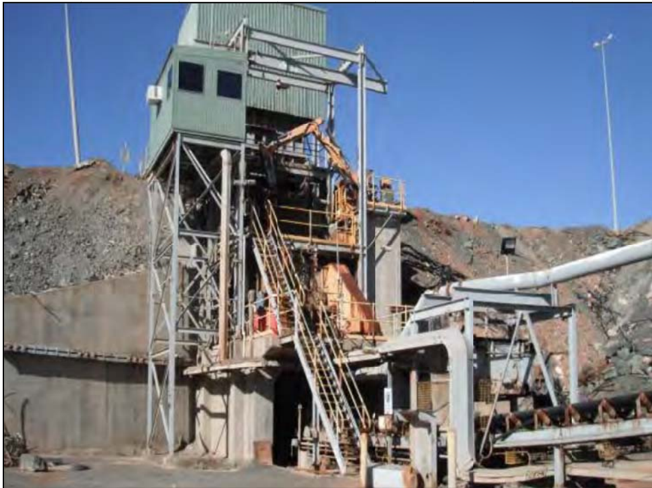
Figure 2: Black Swan primary crushing circuit
