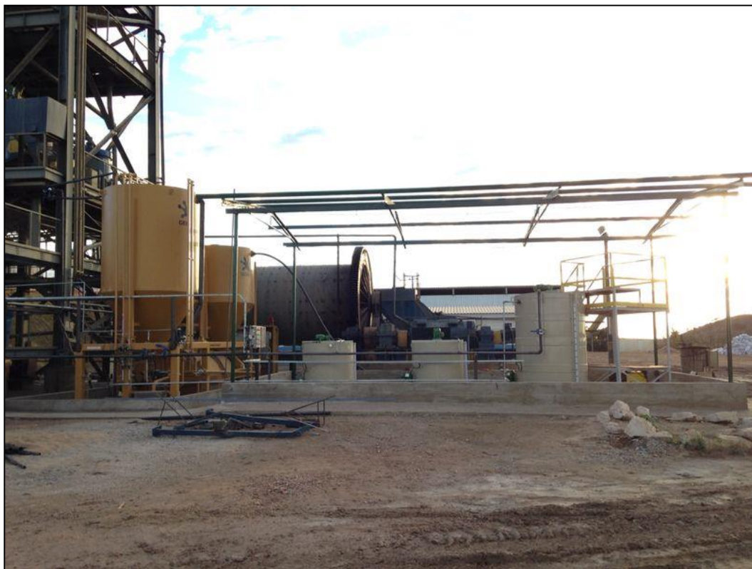
In-Line Leach reactor (yellow) with gravity circuit on left, detoxification tanks on right, and ball mill in background
