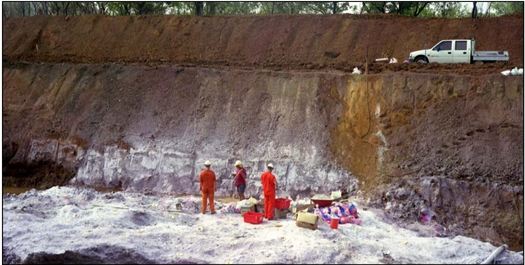
Figure 5 Test mining of magnesite at Winchester deposit. Crew standing on top of the magnesite mineralisation. Deposit has only few meters of overburden and a low strip ratio.
