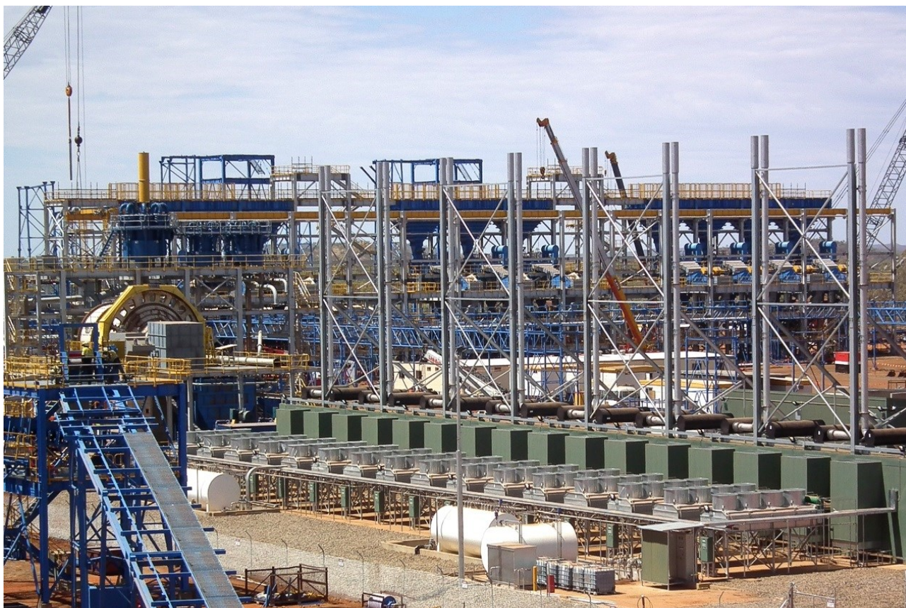
Figure 22: Power Plant (right), Ball Mill (left) and Gravity Jig Building in background,
