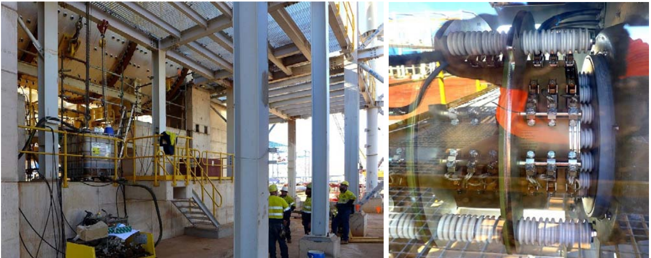
Figure 32: Pipe-bridge structure (top image); Ball Mill lining being installed (middle image); pre-start meeting at Ball Mill (bottom left) and shielded high-voltage transformer at the Ball Mill drive train (bottom right)
