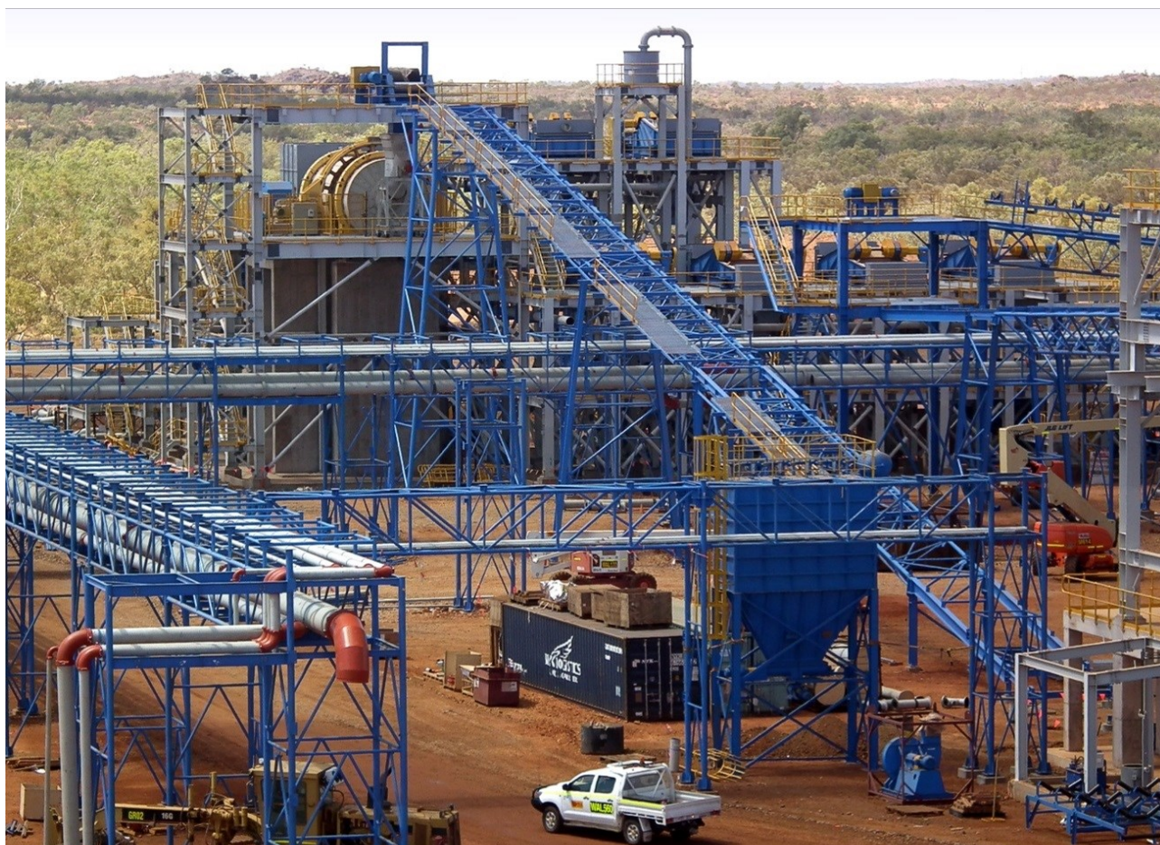
Figure 26: Transfer infrastructure connecting the HPGR to the scrubber.
