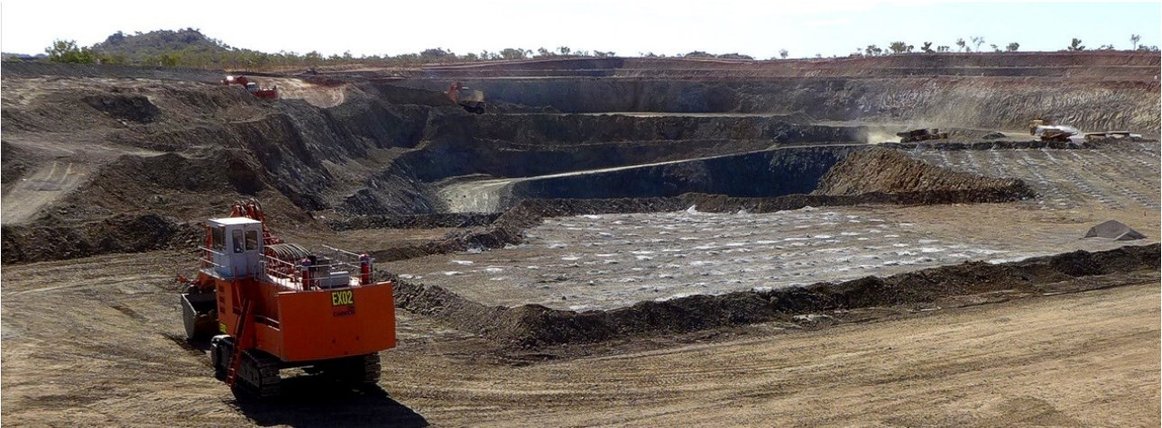
Figure 45 (three stages of the LM Pit); LM2 Pit taking shape around the smaller LM1 Pit (middle distance) and the walls of the final Pit (LM3) can be seen in the far distance.
