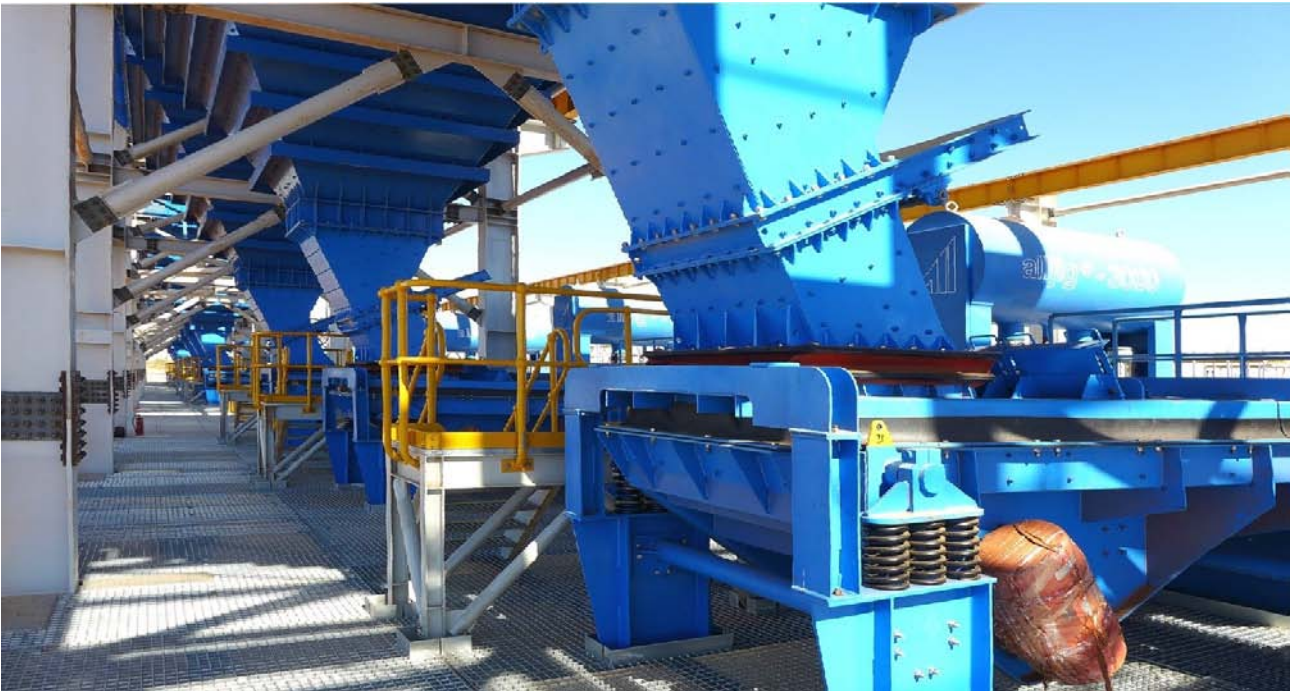
Figure 28: Gravity Jig Building - Top image; feed bins (top), screen on middle floors and pump-boxes on ground floor. Feed chutes into ore jigs.
