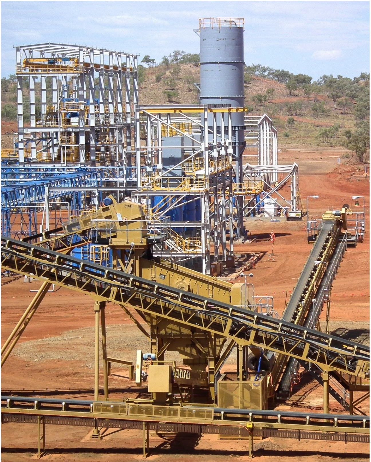
Figure 27: Conveyors from the Crushing Circuit (foreground), Magnetic Separator (middle distance) and Thickener/Filtration circuits in the background.
