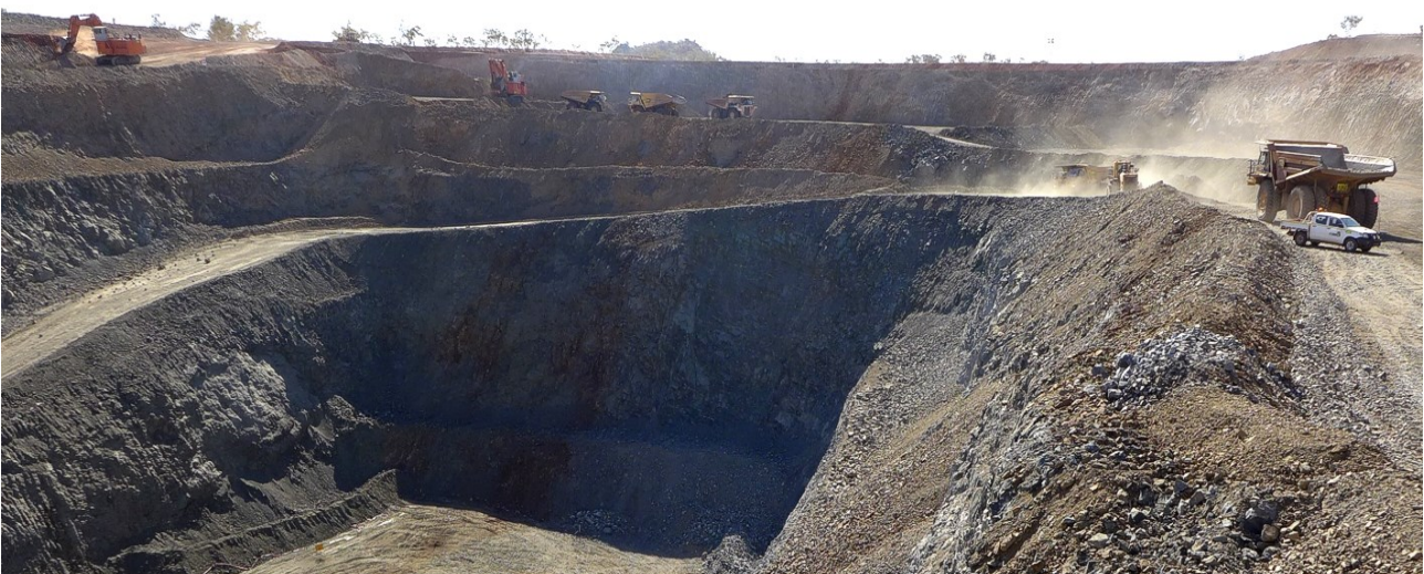
Figure 46: LM1 Pit (foreground) is temporarily closed off as mining on the south-west wall of LM2 (left of image) removes recently blasted waste to make access safe. Mining at the north-west of LM2 can be seen in the background and to the right, concurrent mining of waste areas also in LM2.
