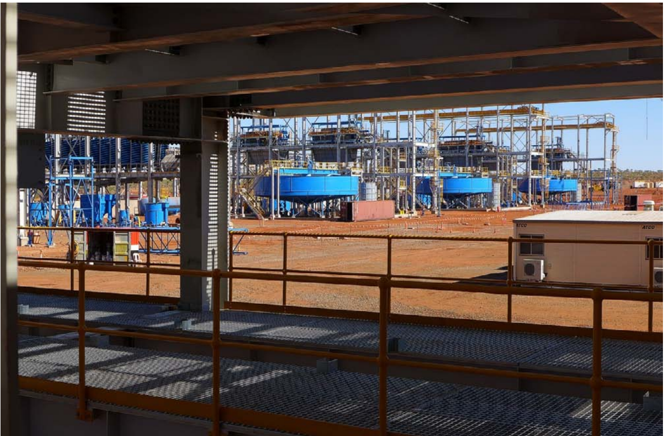
Figure 30: Flotation Cells (top image) and in background; Spirals (left) and Thickener/Filtration circuits (right three structures)
