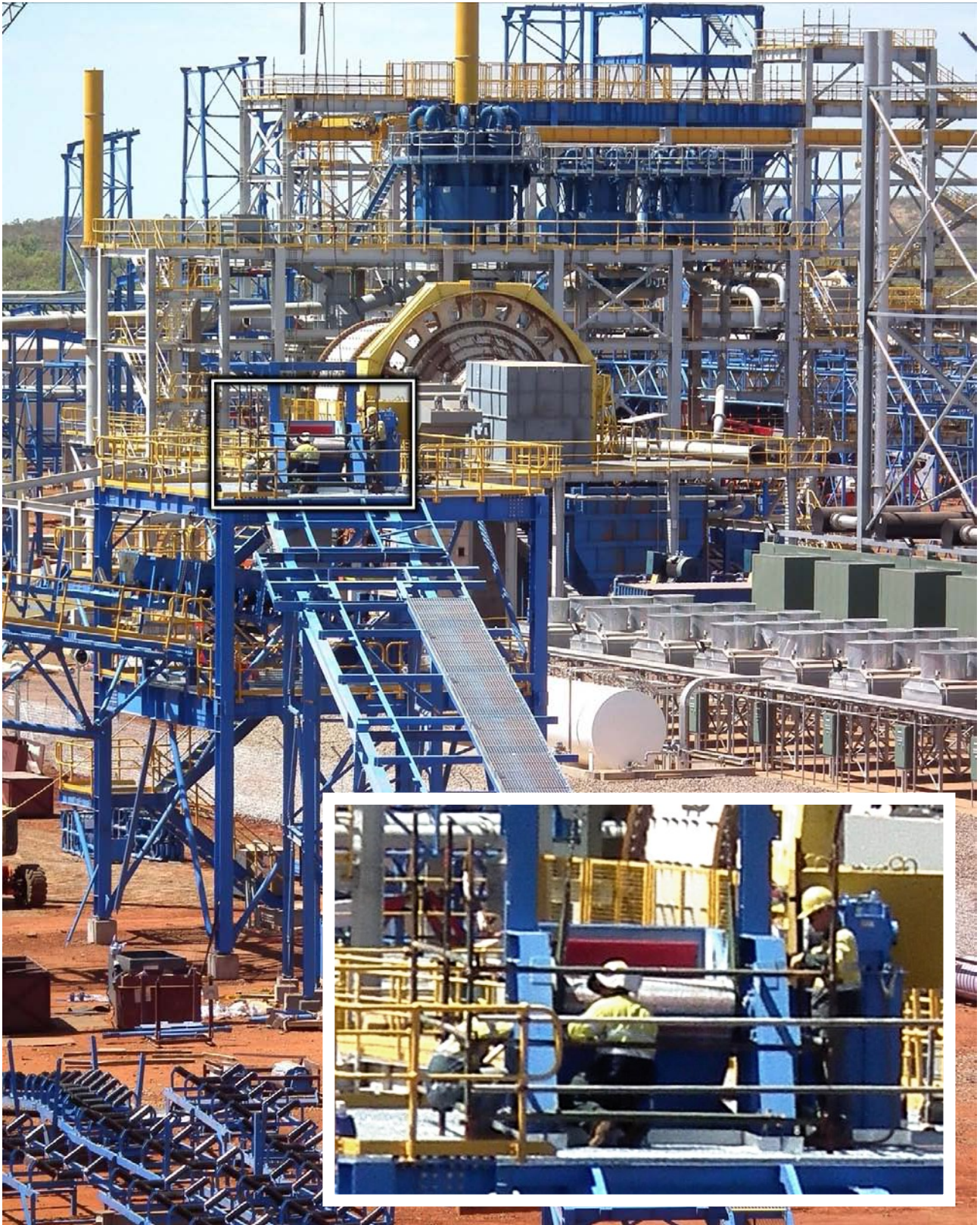
Figure 37: Rocklands Process Plant - major components installed and structural completion underway. Inset of workers helps give scale - they are clearly dwarfed by the infrastructure.
