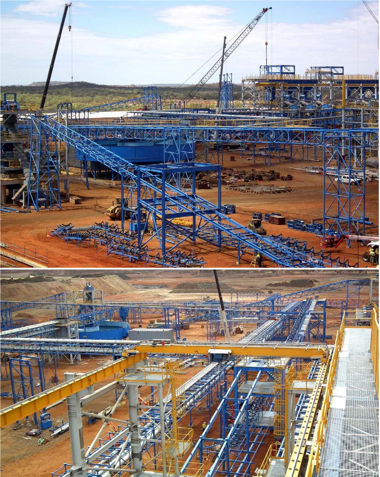
Figure 38: Transfer infrastructure pipe bridge connects various circuits and components of the processing plant including the HPGR, Scrubber, Gravity Thickener and Gravity Jig Building. Workers are dwarfed by the size of the process structures.
