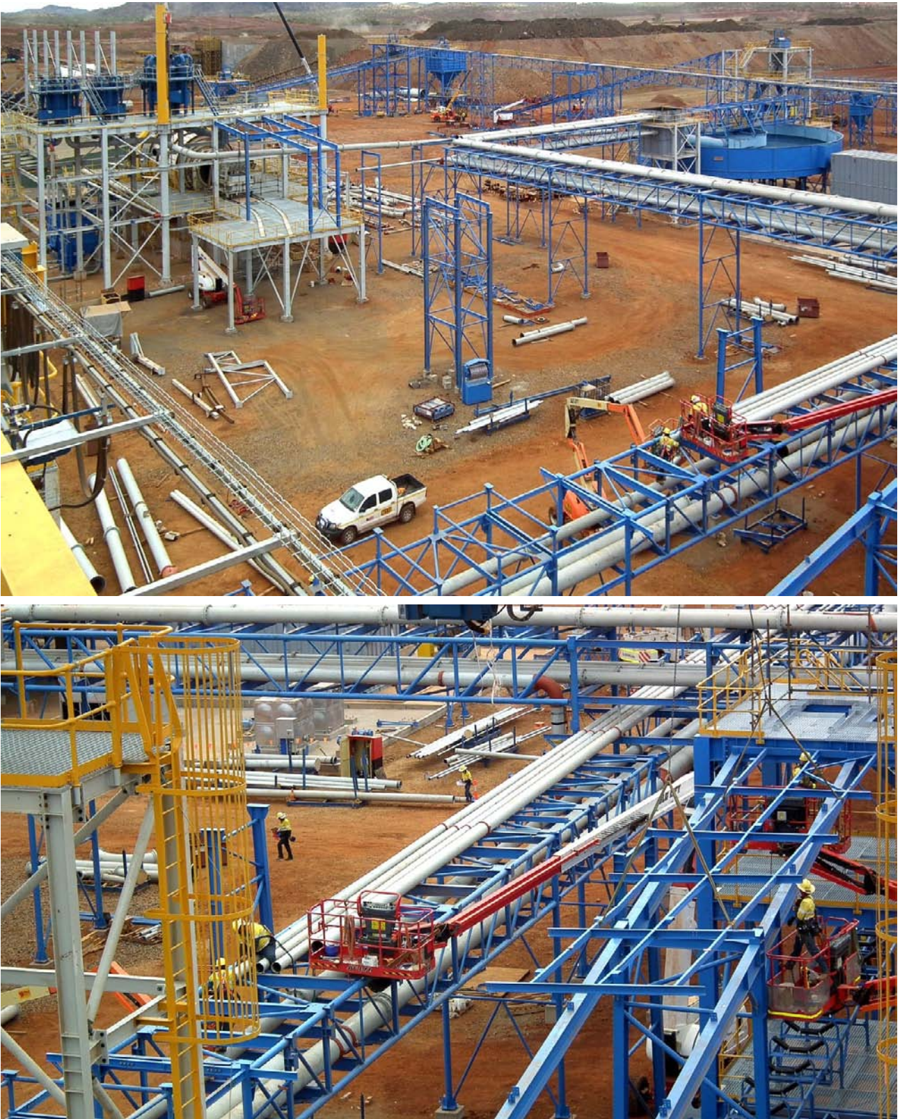
Figure 39: Transfer infrastructure and pipe bridge connects various circuits and components of the processing plant including the HPGR, Scrubber, Gravity Thickener, Gravity Jig Building and Ball Mill. Workers are dwarfed by the size of the process structures.
