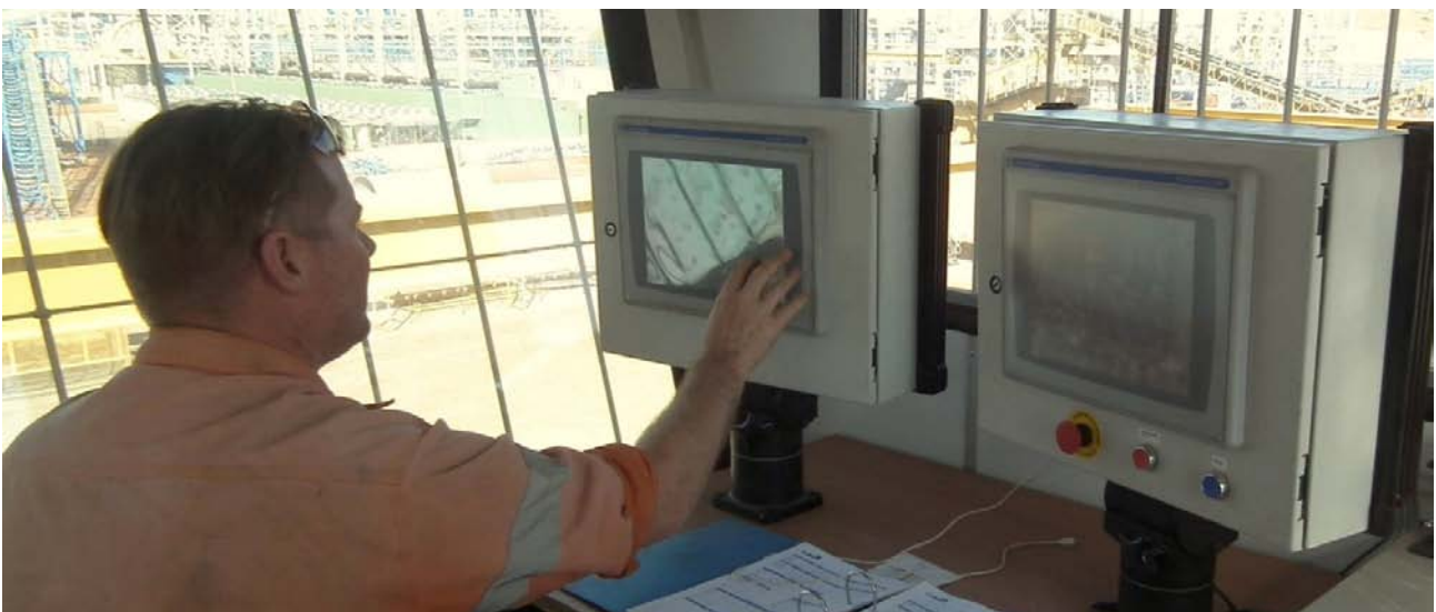
Figure 4: Crusher Operator Bevan Nolan checks settings on the Crusher Control Panel
