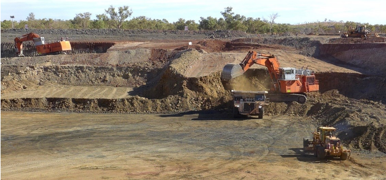
Figure 50: Mining ore and waste on the north-west shoulder of LM2 pit after blasting. The darker ore zones are clearly visible on the pit floor.
