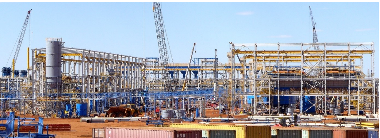
Figure 40: Rocklands Process Plant - major components installed and structural completion underway. From top to bottom; Pipe-bridge infrastructure connecting the HPGR feed (right) to the Scrubber (left), Gravity Thickener and below image shows Flotation Building (left), Gravity Jig in far background and Thickener/Filtration circuits (right).
