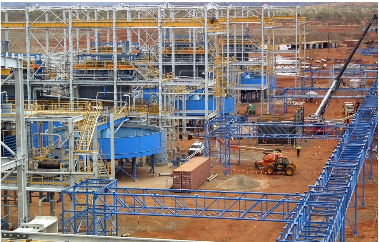
Figure 23: Bank of three Thickener/Filtration Circuits as viewed from the Gravity Jig Building.
