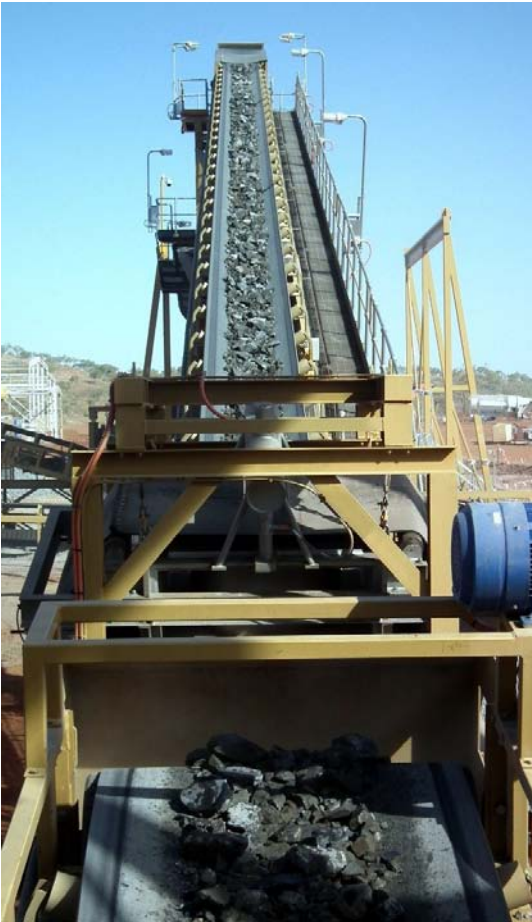
Figure 3: Conveying ore from the Primary Jaw Crusher to the screen above No 1 Rolls Crusher
