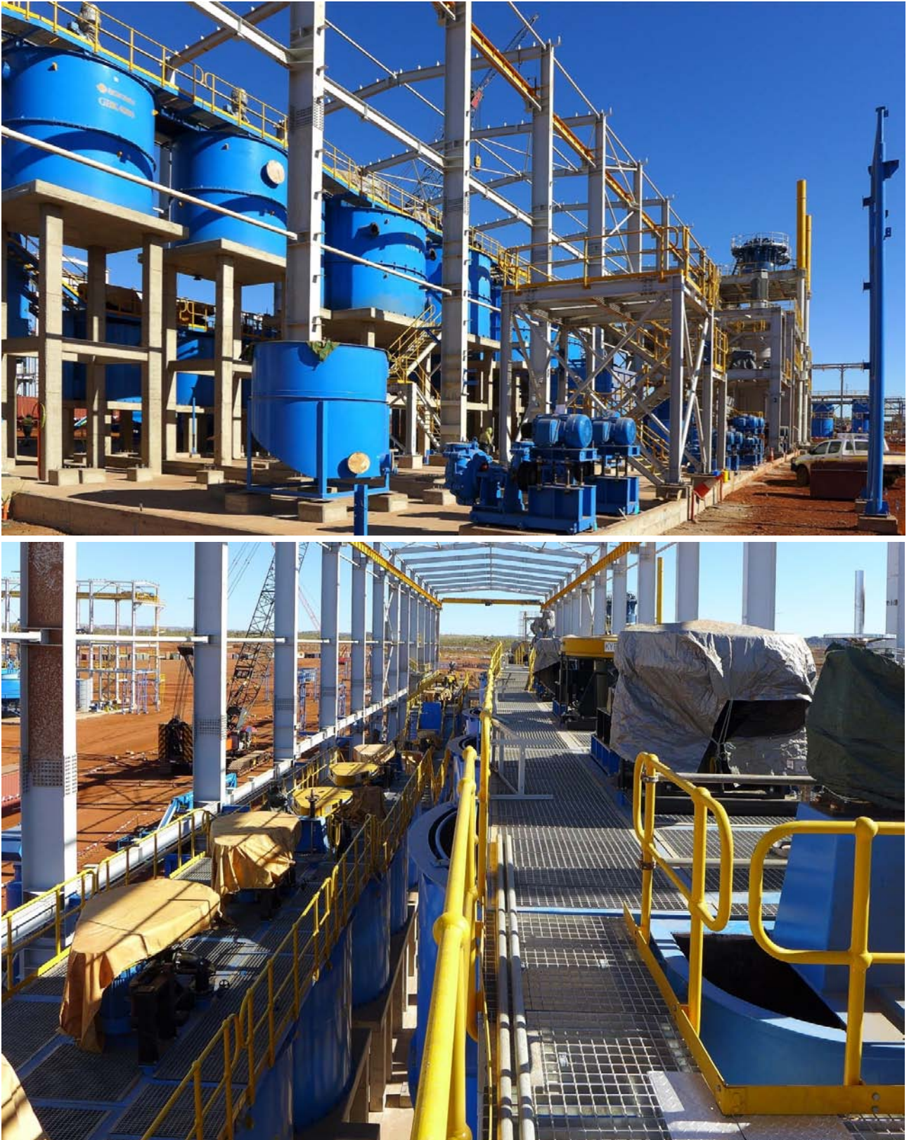
Figure 31: Flotation Cell building - flotation cells (top) and cell agitators (bottom)
