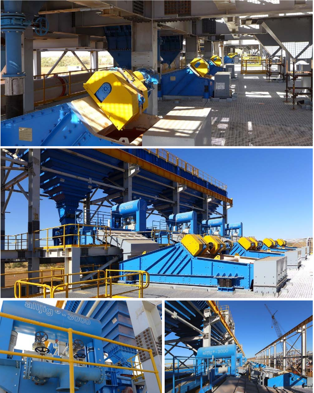
Figure 33: Gravity Jig Building - from top to bottom; native copper metal screens, feed bins and light screens and continuous alljig® units (left and right)
