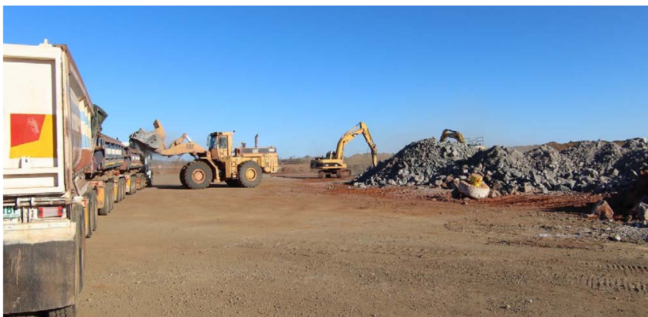
Figure 6: Contractor loading road trains with Rocklands primary ore ready for shipment to EHM processing plant
