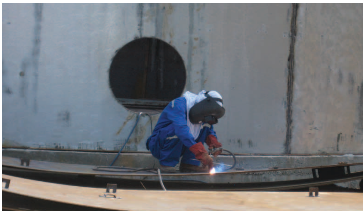
Welding of large storage tanks at the Lubuk Mandi Gold Mine, Malaysia.
