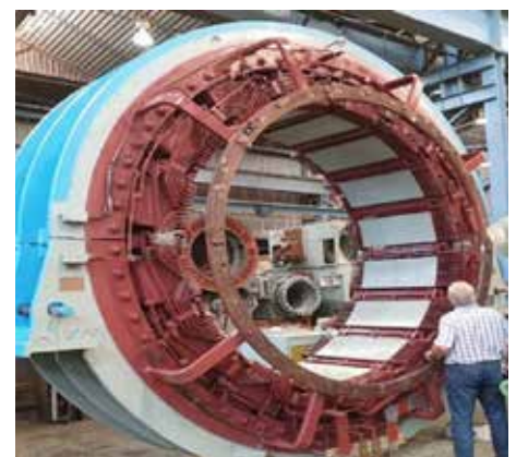
Fully Reconditioned Stator at Marthinusen & Coutts
