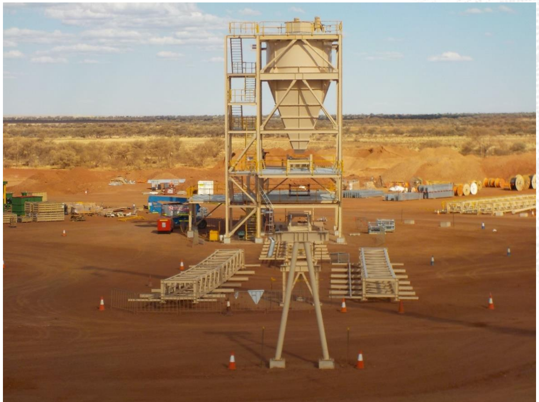
Figure 8: In Feed Transfer Crushing Station
