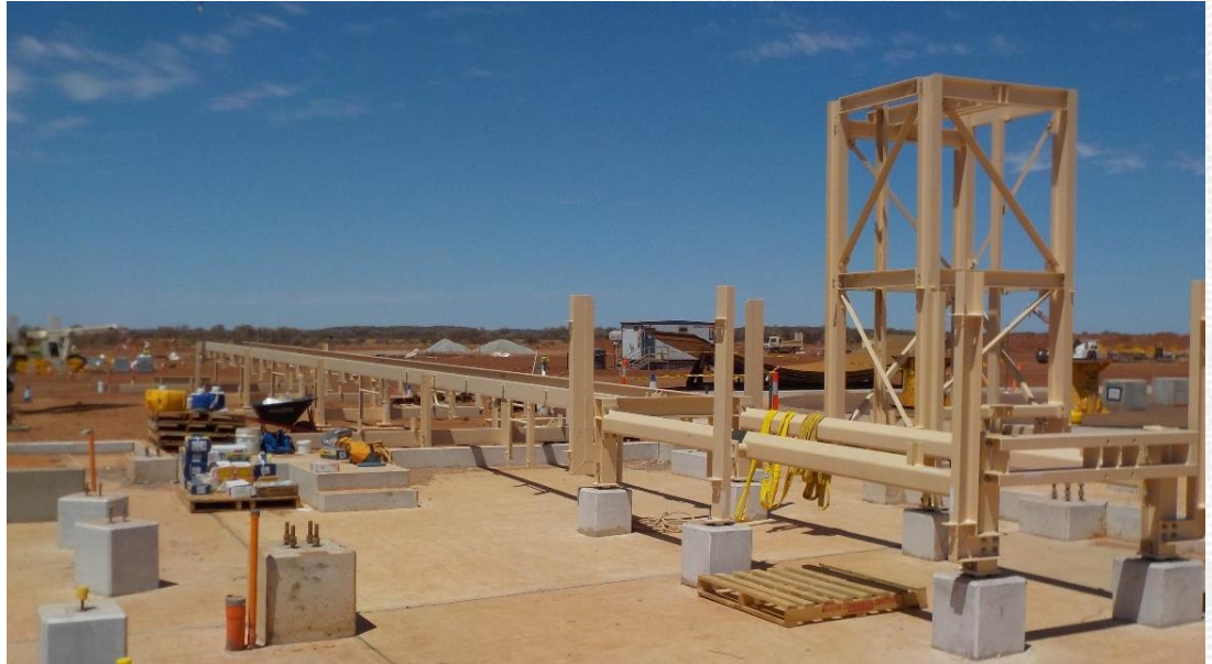
Figure 7: NaCl waste conveyor structure and gravity take up tower
